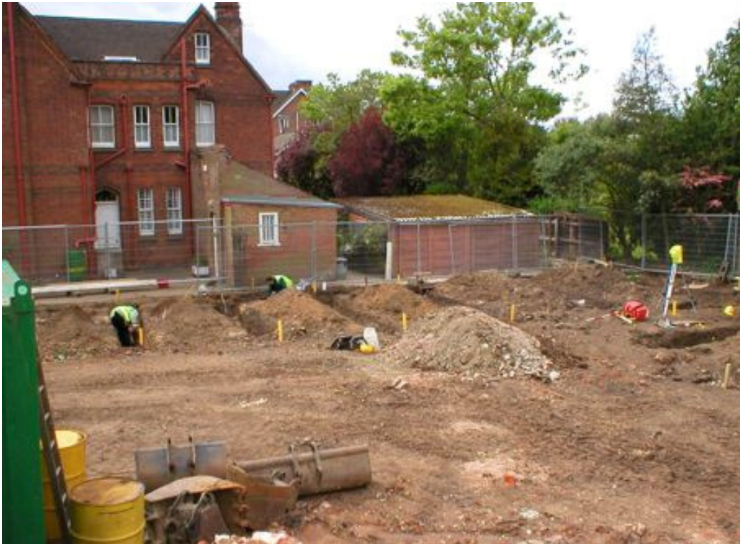
Plate 3: the site during excavation, view west, looking towards 21 West Lodge Road (frame ref: 2583)
