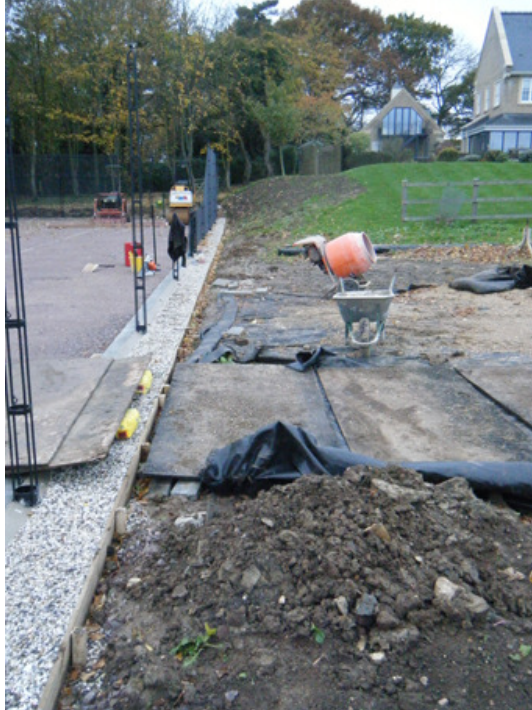
Photograph II Side of tennis court after fence-posts erected. Upcast visible by each post. Shot taken facing west.
