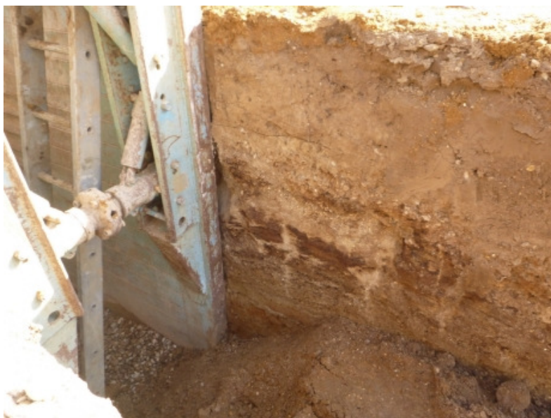
Photo. 5: Deep section in drain trench in north-western part of the site, height of cleaned section approximately 1.8 m (view south-east).
