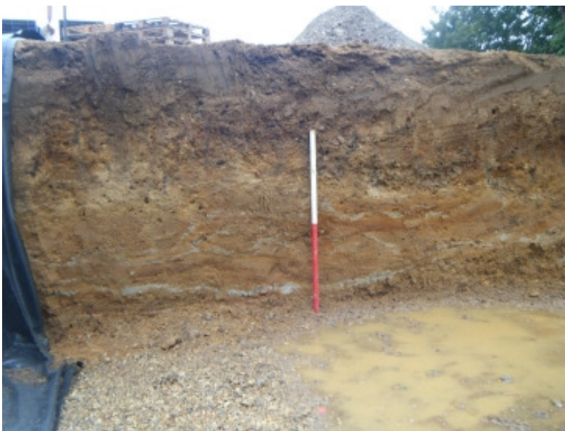
Photo. 2: Section of deposits in trench for attenuation tank, modern gravel spread in foreground (view south-west).
