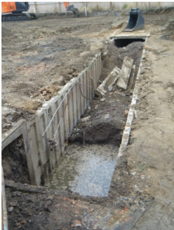
Photo. 6: Air-raid shelter, entrance in bottom left-hand corner; note: water is surface run ponding in base not groundwater (view north-west).
