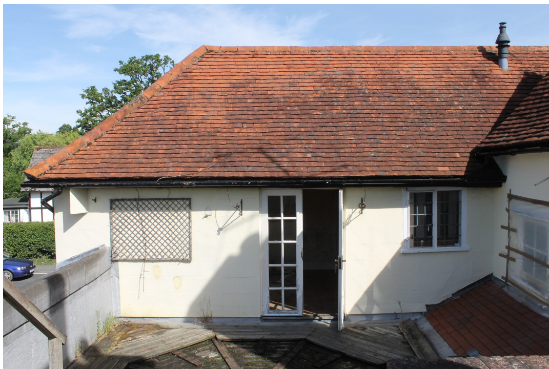
Photograph 7 South-east elevation of the first floor to the 16th-century cross-wing with a surviving 16th-century casement window to the right - view north-west.
