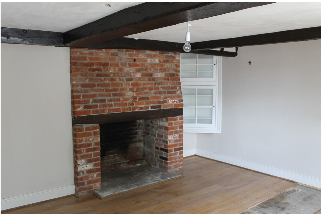
Photograph 18 Inserted 19th-century fireplace with modern fire surround in GF2 and 19th-century corner cabinet – view west.
