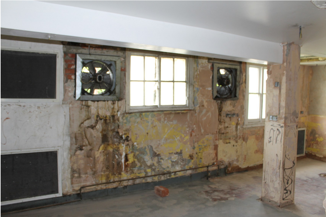
Photograph 19 Interior of 19th-century single-storey extension on north-west side of GF3 with possible surviving 16th-century storey post and girding beam concealed beneath modern materials – view north.
