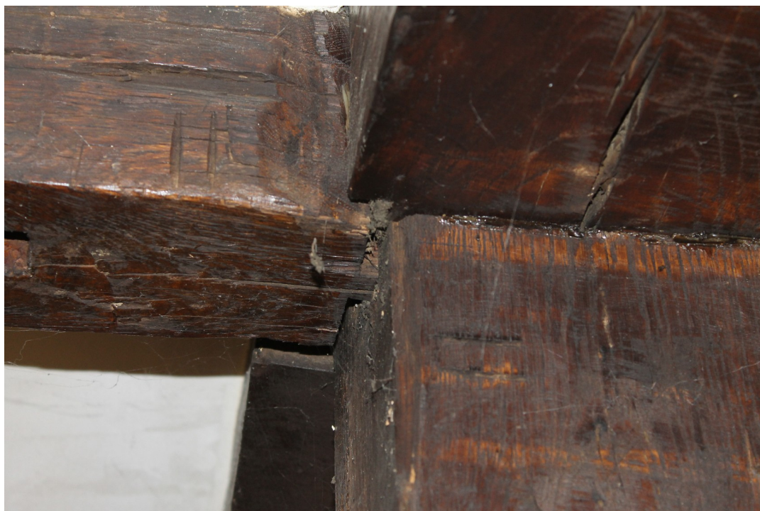
Photograph 13 Detail of chiselled carpenters' marks on bridging beam and post in GF1.
