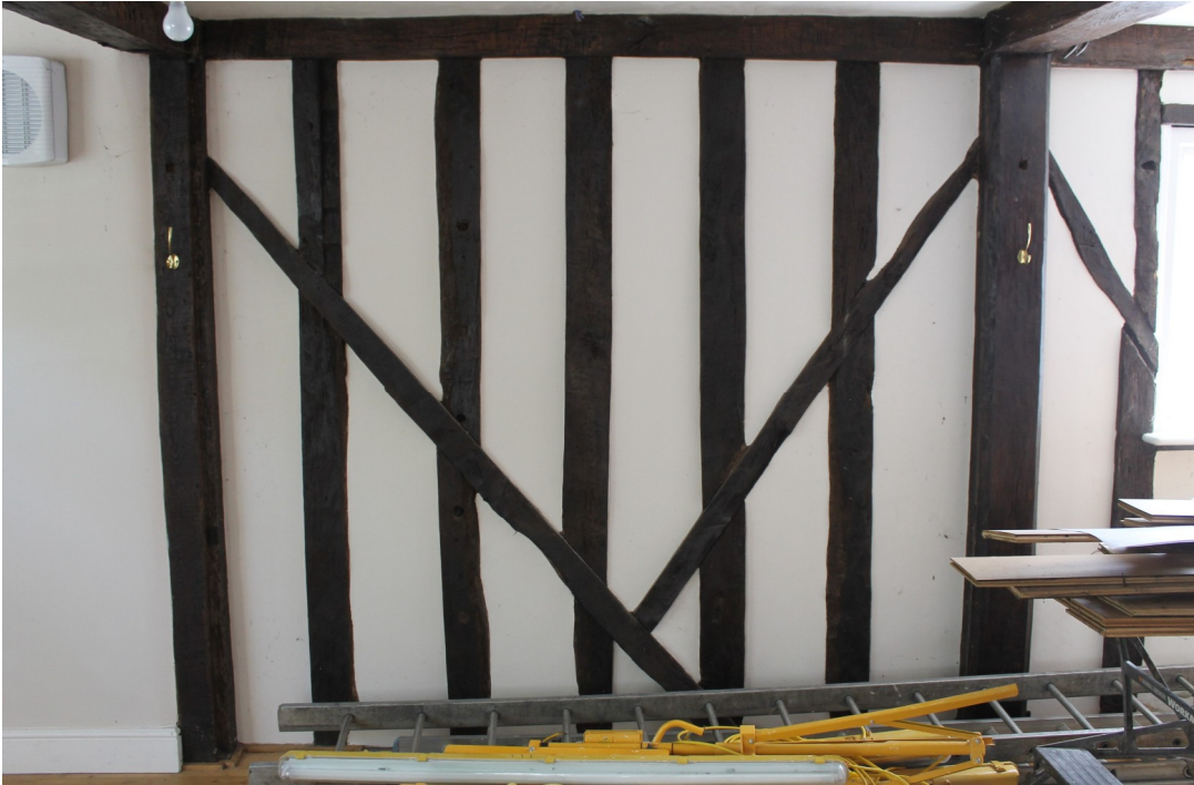
Photograph 11 Original 15th-century studs in south-east wall of GF1, with later internal bracing - view south-east.
