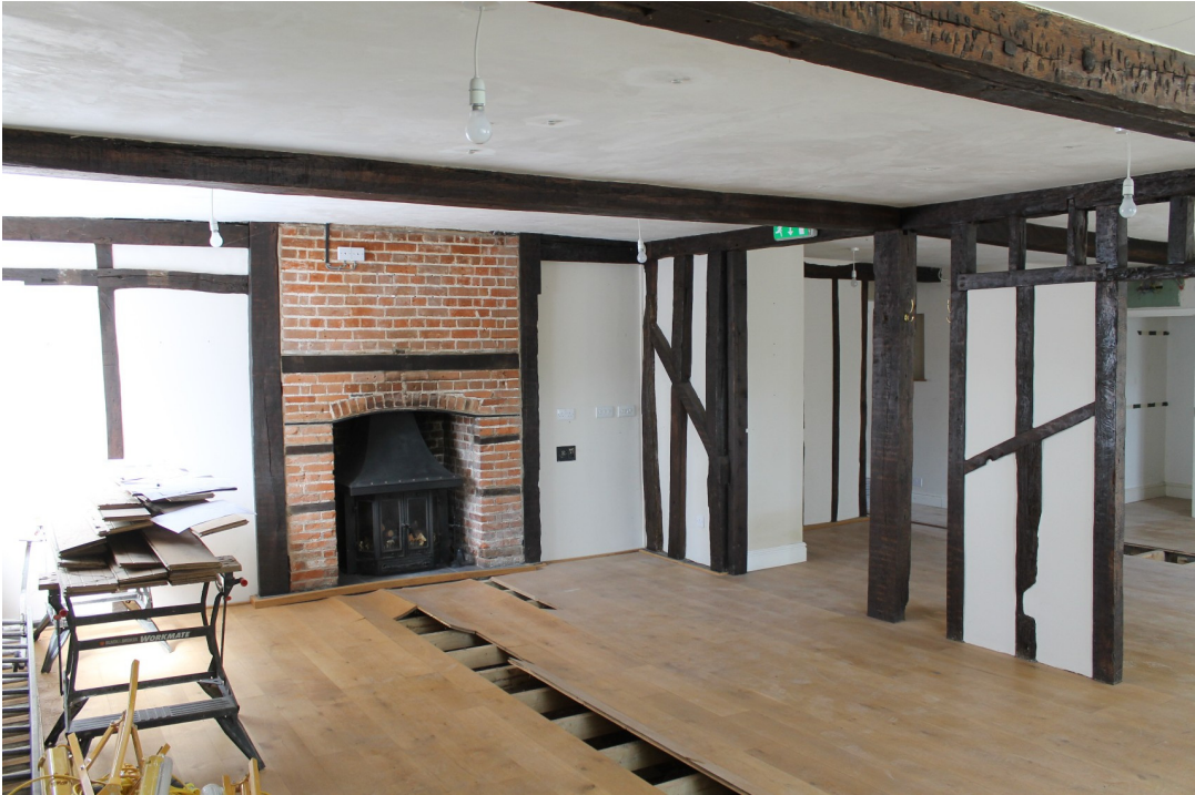
Photograph 9 Interior of GF1, 15th-century main range with inserted 18th-century fireplace and repositioned stud work - view west.
