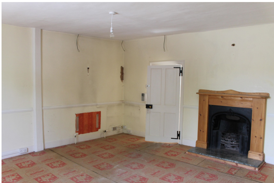
Photograph 21 Interior of FF1 with 15th-century storey post to the left and 18th-century cast-iron register grate to the right – view south.
