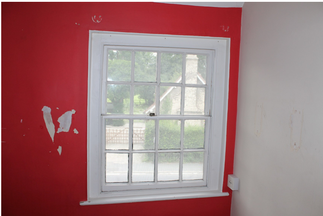
Photograph 30 18th-century sash window in FF7 with 20th-century stud wall to the right – view north-west.
