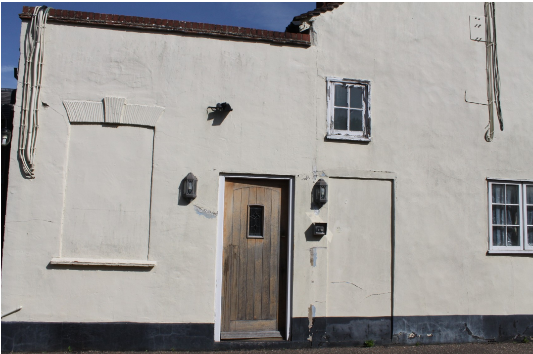
Photograph 6 South-east elevation of the 1923 extension with blocked window and an earlier blocked doorway to the 18th-century staircase on the right - view north-west.
