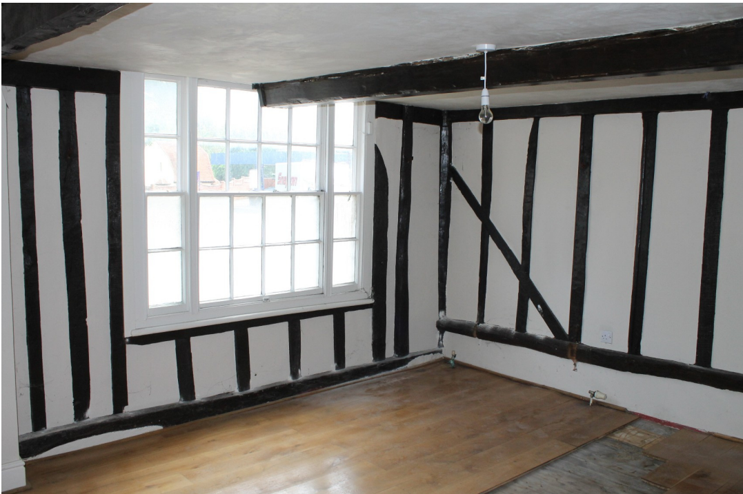
Photograph 16 19th-century sash window with margin lights inserted into north-east framing of the 18th-century extension to the 16th-century cross-wing (GF2) – view east.
