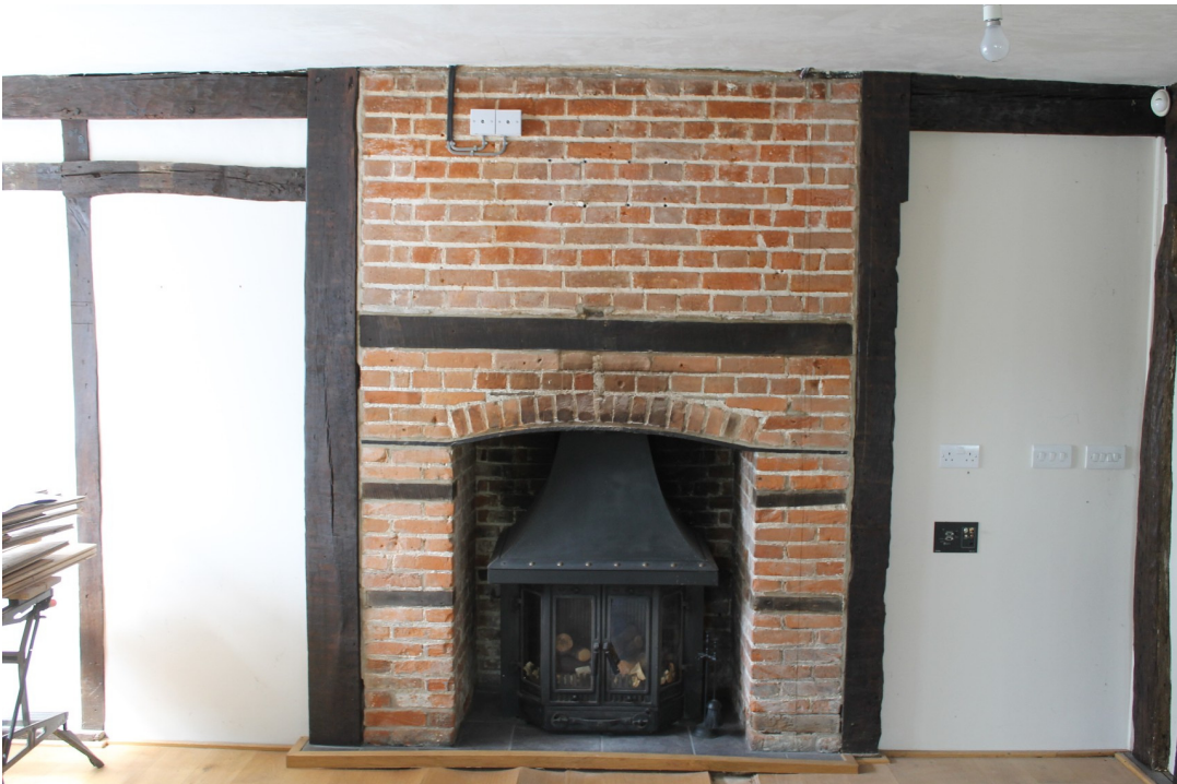
Photograph 12 18th-century fire surround in GF1 with blocked access to the external staircase on the left - view south-west.
