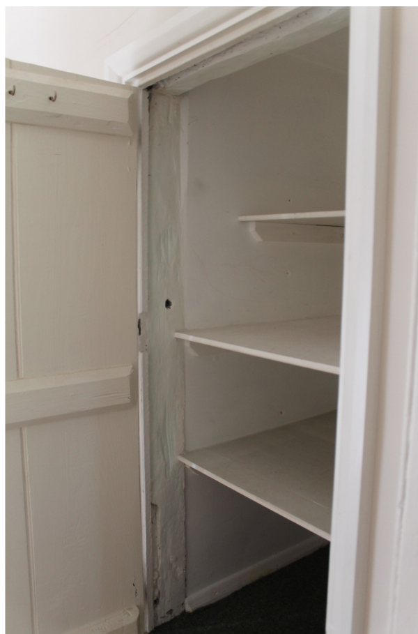
Photograph 24 Interior of small cupboard built against chimney stack on landing outside FF1 – view west.
