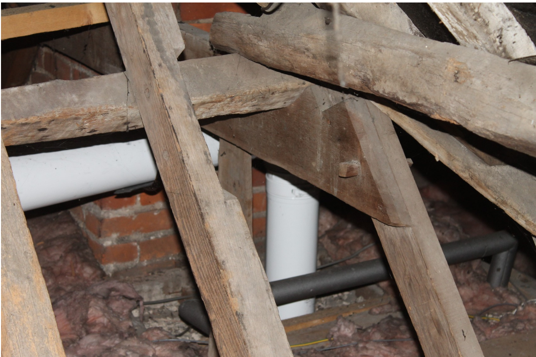
Photograph 34 Purlin of main range supported on purlin above 16th-century cross-wing – view north-west.
