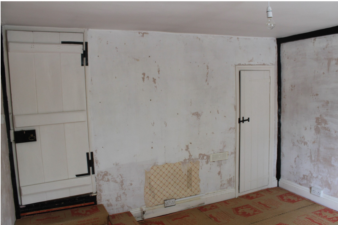
Photograph 26 Interior of FF4 showing the front of the 16th-century cross-wing (timber frame obscured by modern plaster), with the cupboard to the right – view west.
