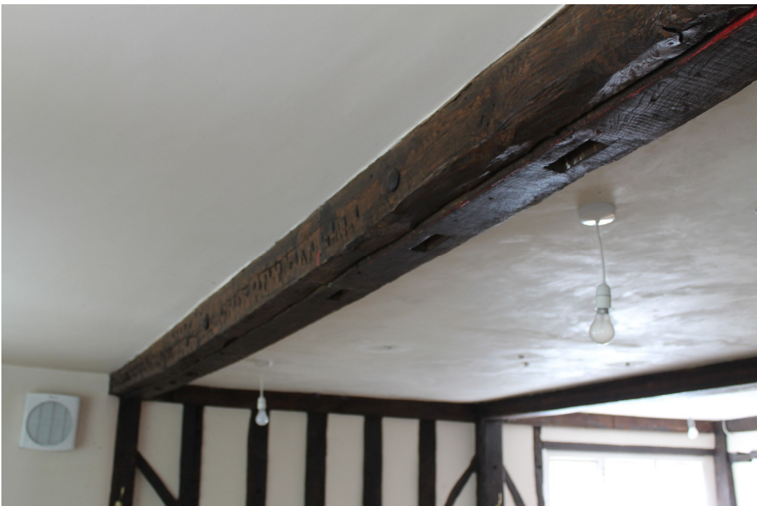
Photograph 10 Exposed mortises in underside of 15th-century beam in GF1 with strengthening beam bolted to the external face – view south.
