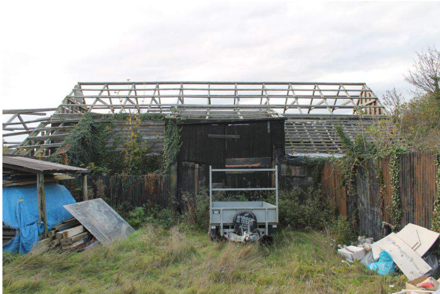
Photograph 1 North-east elevation of threshing barn and lean-tos (on the right). Photograph taken facing south-west.
