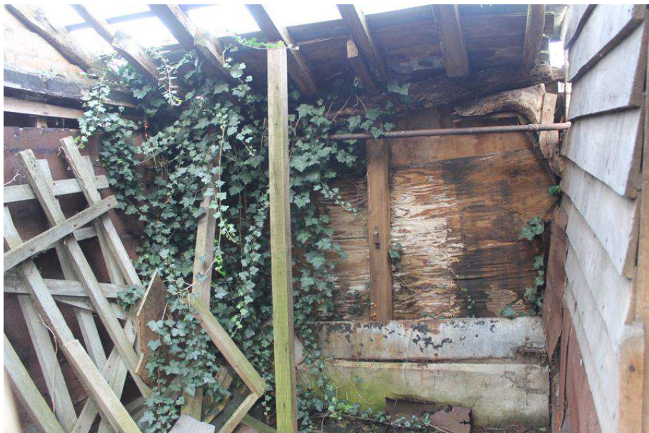
Photograph 24 Interior of southern lean-to, showing damaged structure, knee brace and inserted concrete plinth. Photograph taken facing north-east.
