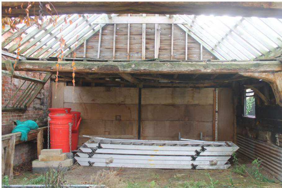
Photograph 30 Bay 3 of cow house, showing tie-beam and first-floor. Photograph taken facing south-east.
