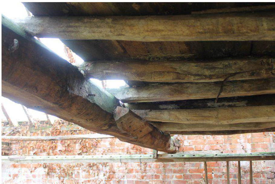
Photograph 36 Shot showing first-floor joists laying on southern tie-beam. Photograph taken facing north-east.
