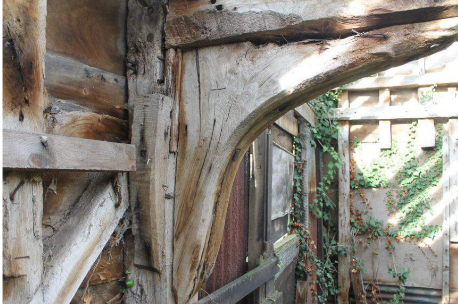
Photograph 33 Knee brace supporting western end of northern tie-beam in cow house. Carpenter's mark "X" visible. Photograph taken facing west.
