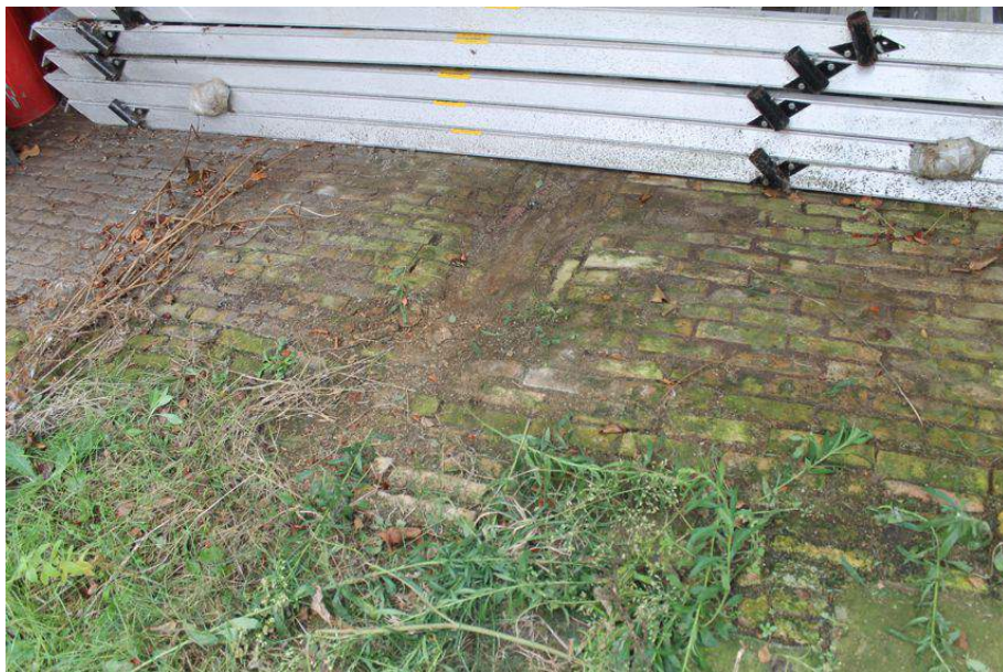
Photograph 34 Detail of surviving brick floor in Bay 3. Drainage channel visible. Photograph taken facing south-east.
