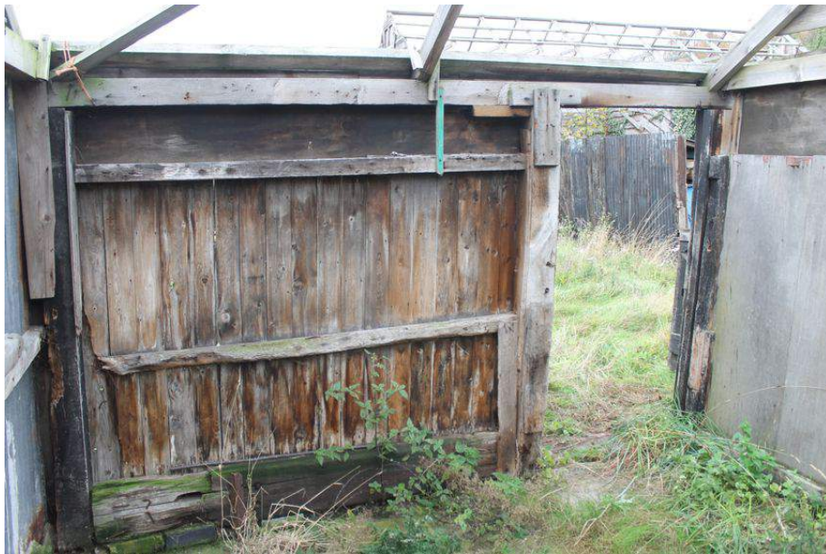
Photograph 42 Interior of stable, showing use of hand-sawn and machine-cut timbers. Photograph taken facing south-west.
