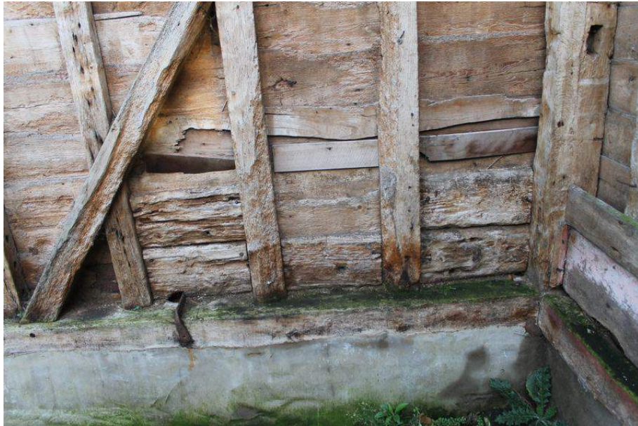
Photograph 10 Detail of wooden nogging panels on east wall of Bay 1. Photograph taken facing north-east.
