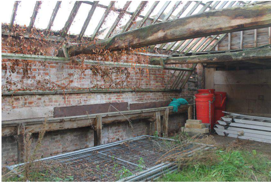
Photograph 29 Interior of cow house, showing red brick wall forming eastern extent of building. Photograph taken facing east.
