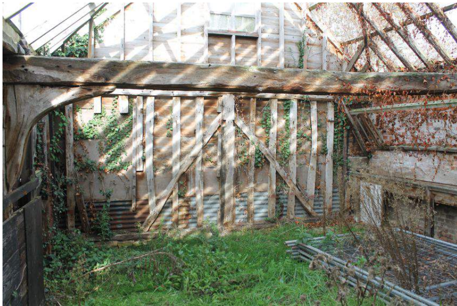
Photograph 31 Interior shot of cow house showing north-east gable end and northern tie-beam. Photograph taken facing north.
