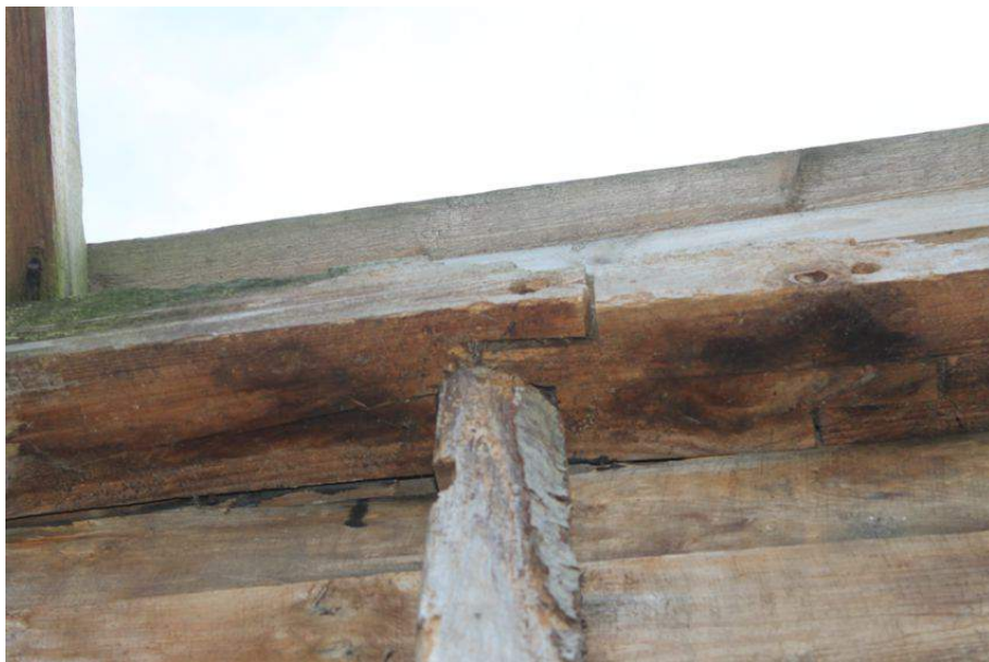
Photograph 11 Detail of scarf joint on western wall-plate of Bay 2. Photograph taken facing west.
