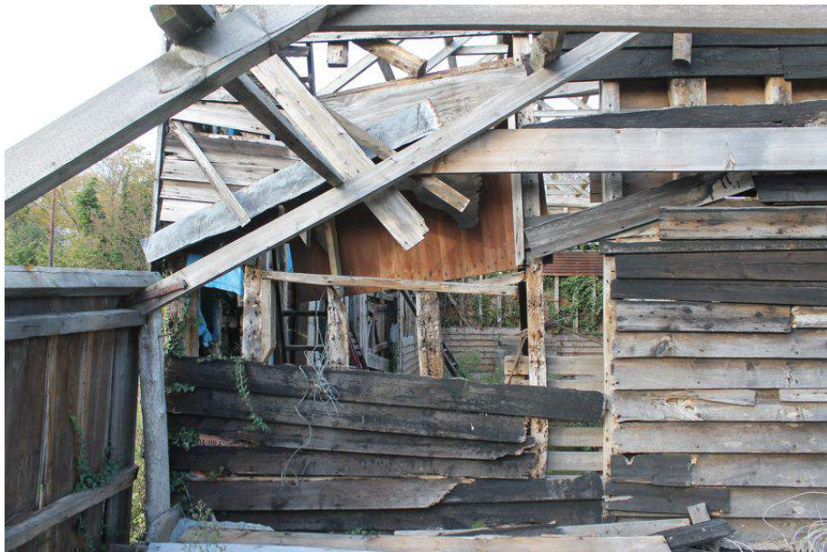
Photograph 3 Detail of damaged timber-frame and missing weatherboarding on south-east elevation of threshing barn. Photograph taken facing north-west.
