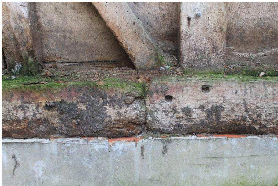
Photograph 9 Detail of scarf joint on southern sill-beam in Bay 1. Photograph taken facing south-east.
