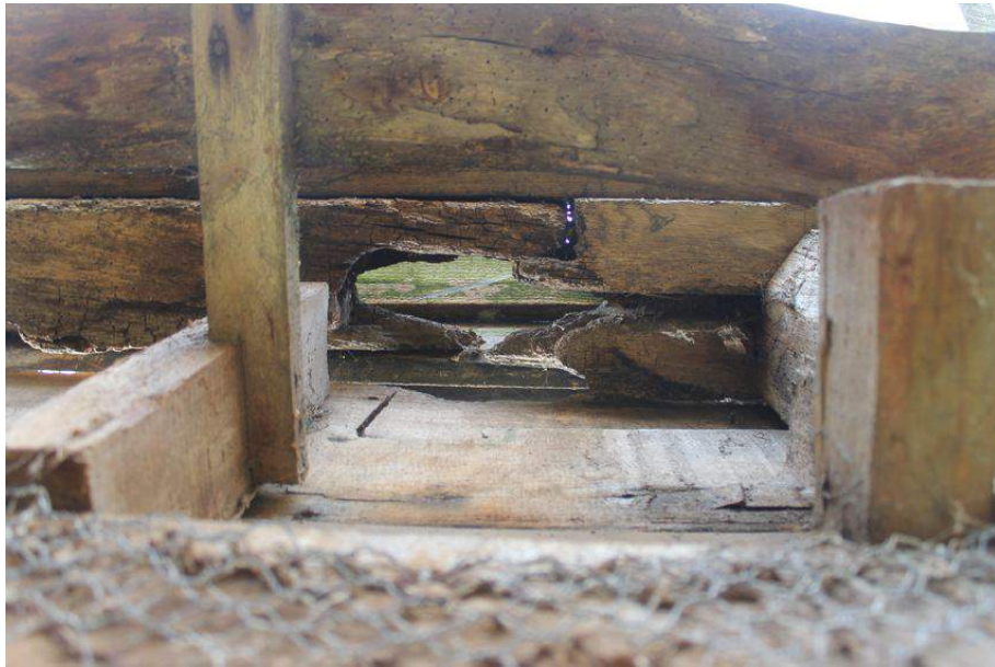
Photograph 35 Detail of degraded joint on western wall-plate in Bay 2. Photograph taken from below.
