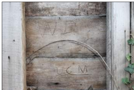
markings on interior of weatherboarding
