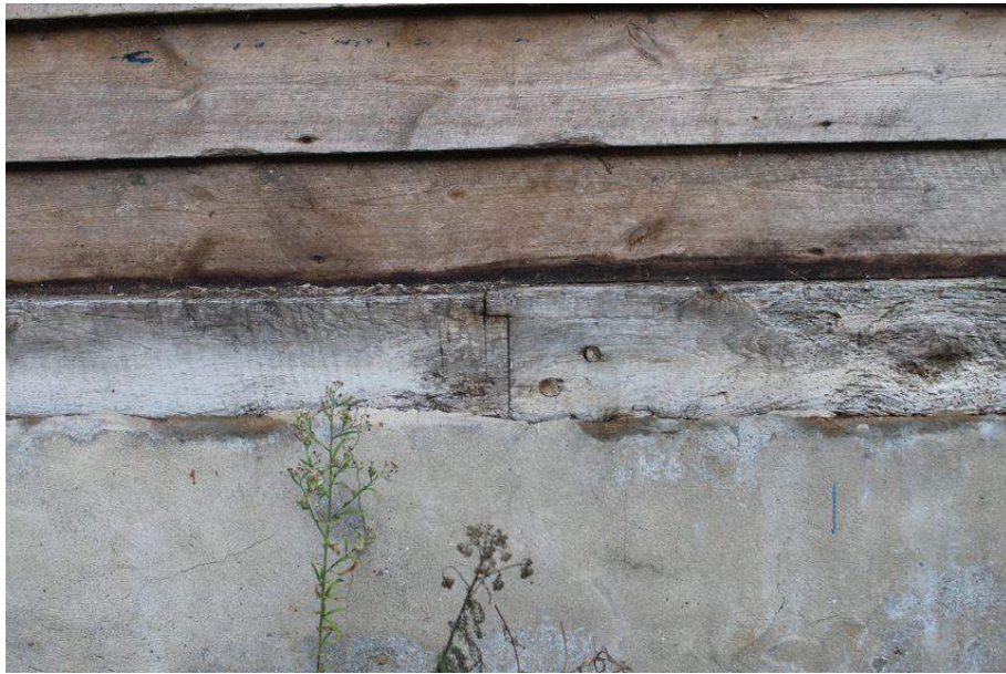
Photograph 15 Detail of scarf joint on eastern sill-beam of Bay 4. Photograph taken facing north-east.
