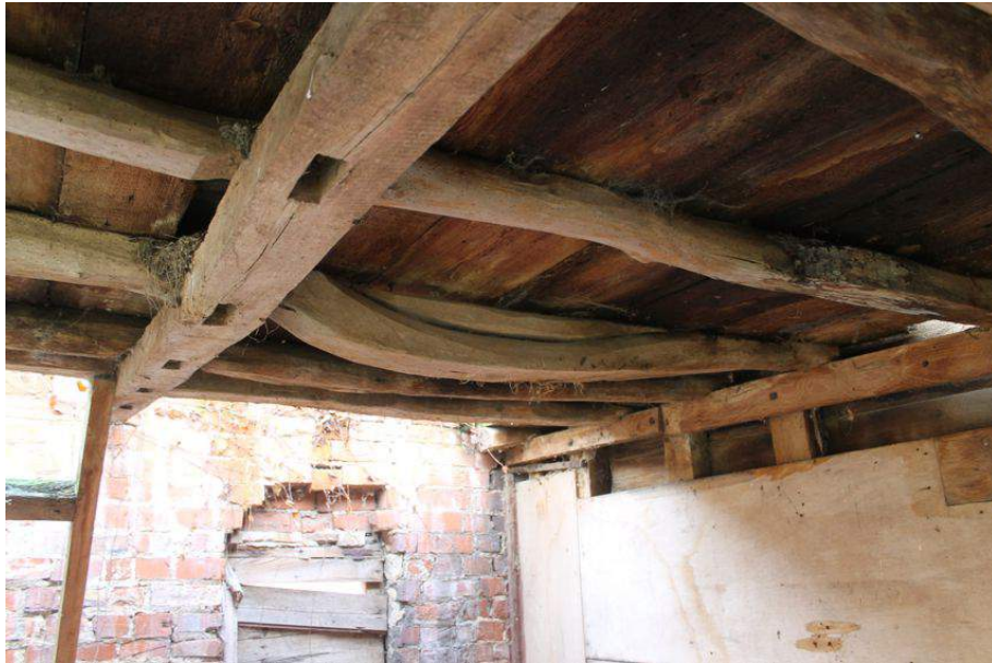
Photograph 37 Underside of first-floor, showing binding-beam with empty mortices and joists being supported on timber nailed to studs on southern wall. Photograph taken facing east.
