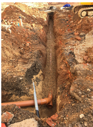
Photograph 1 The trench for a new drainage pipe (photograph supplied by the groundworks contractor), looking east
