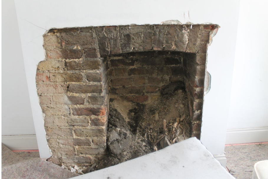
Photograph 14 Exposed fireplace in southern room of main range on first-floor of No 10. Photograph taken facing south-east. An original cupboard survives on the first-floor landing of No 12 (Photograph 15). Although the interior shelves appear to be more recent replacements, the cupboard's four-panelled door is probably original.
