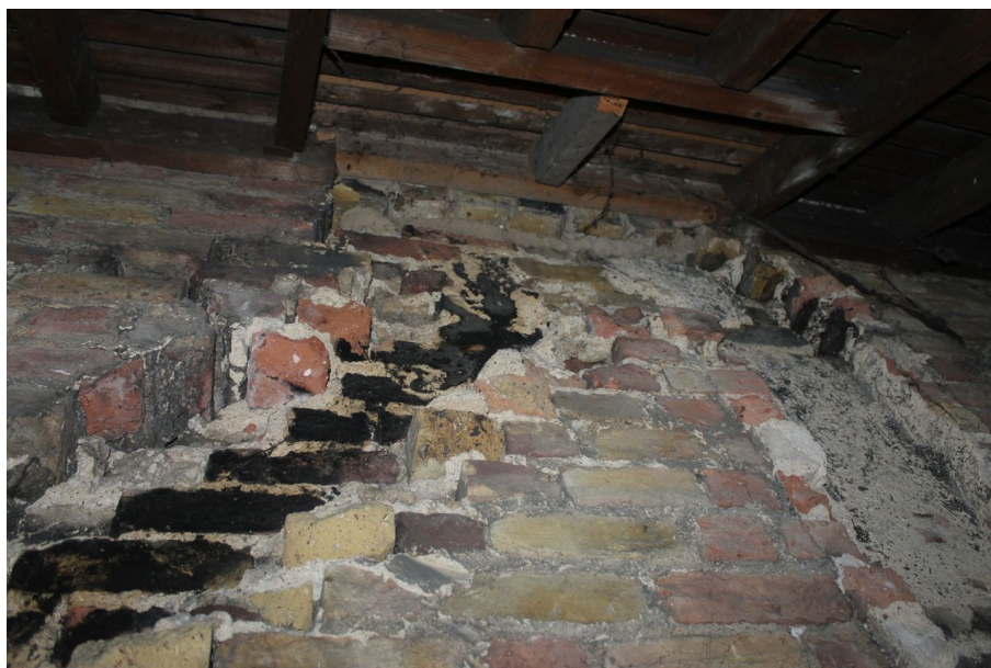
Photograph 13 Remains of chimney in the attic space of No 11's south-west wing. Photograph taken facing south-east.
