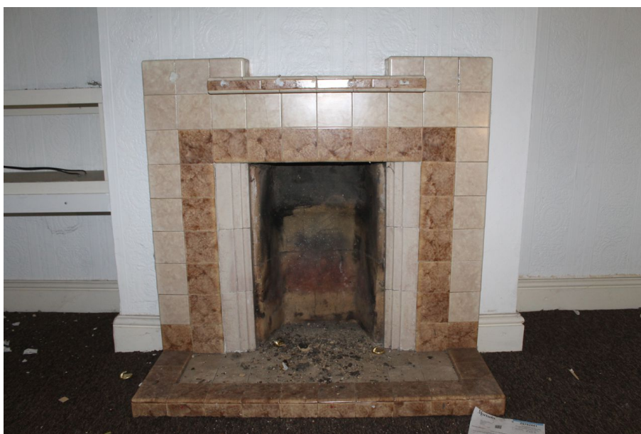
Photograph 9 1930s tiled fireplace surround in living-room on ground-floor of No 12. Photograph taken facing south-east.
