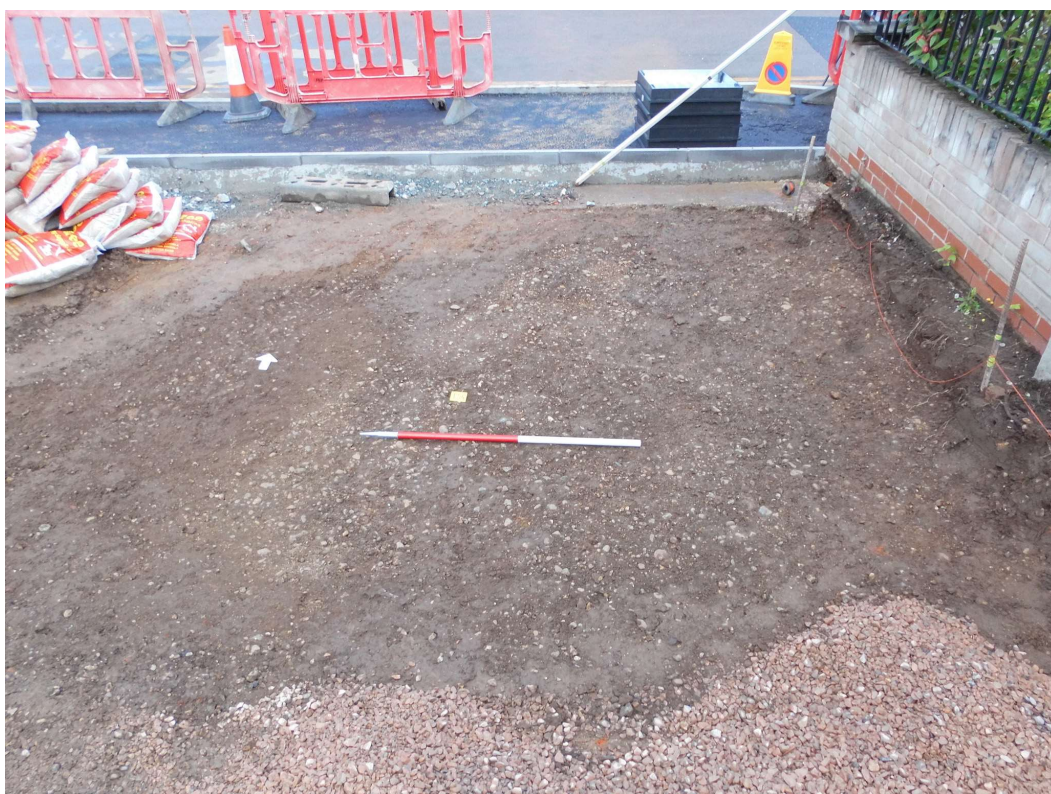
Photograph 19 Ground reduction in the northeast corner of the site revealing metallised road surface WBF54, looking north
