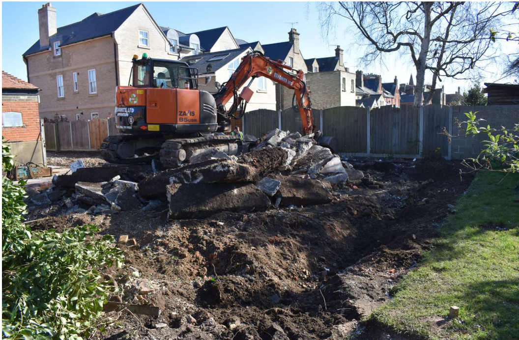
Photograph 5 Southwest corner of the demolished building after the footings and slab had been removed, looking northeast
