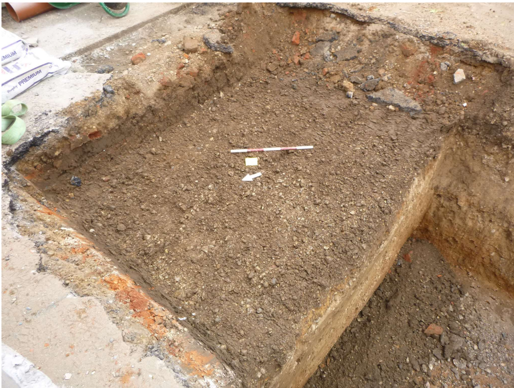
Photograph 18 Metalled road surface WBF54 uncovered during excavation of the inspection chamber, looking southeast
