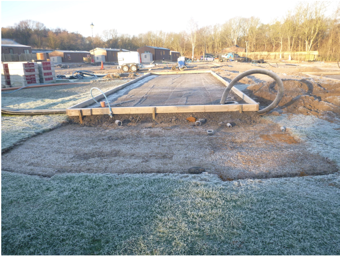
Photograph 4 Example of a built-up foundation pad with drainage set at ground level, looking west.
