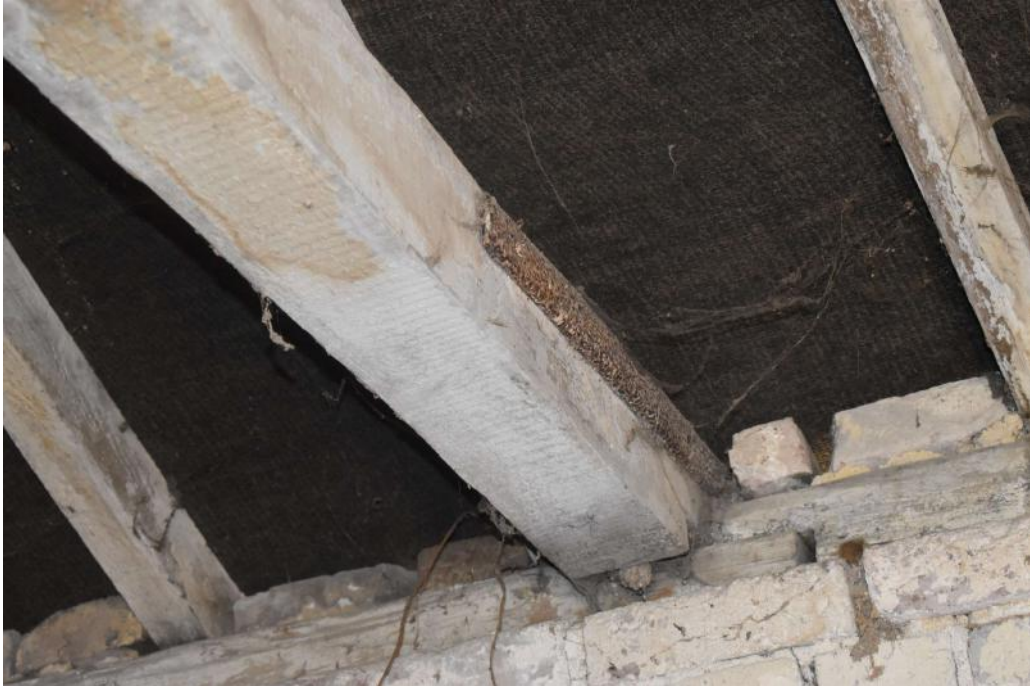
Photograph 35 Interior of Pond Barn, detail of iron tie-beam strap and side-halved scarf joint in wall-plate, south-west wall (building 7). Photograph taken facing south-west.
