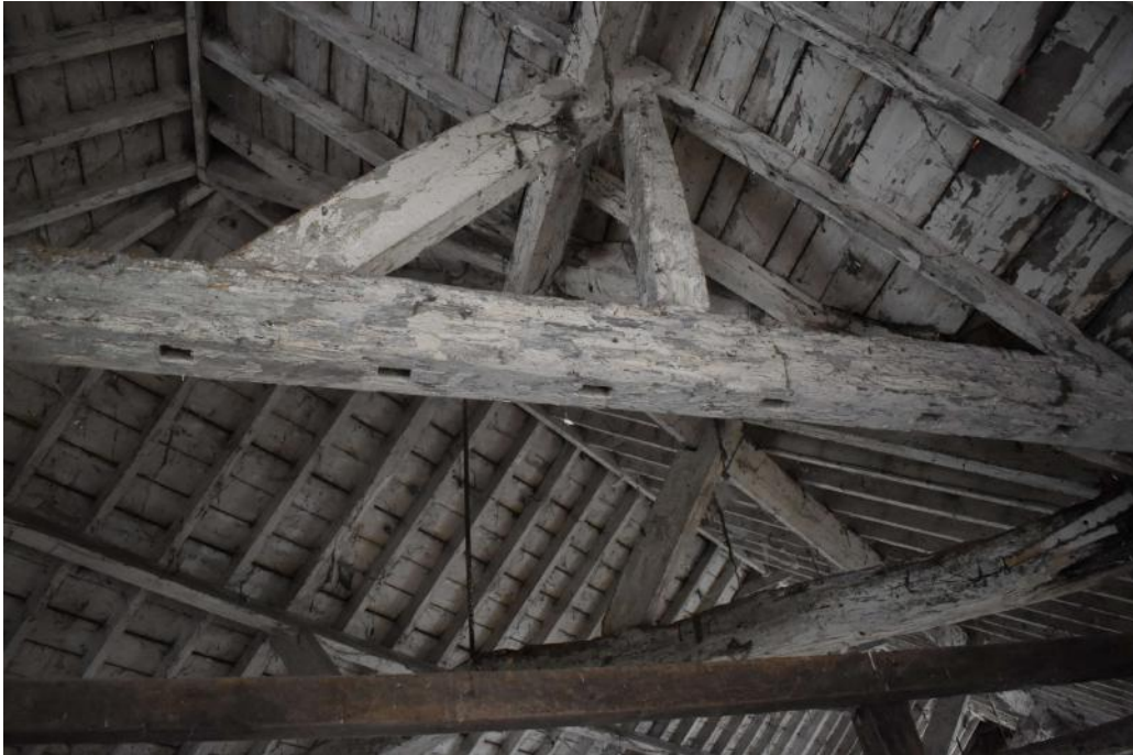
Photograph 24 Interior of Road Barn, detail of empty mortises in tie-beam (building 3). Photograph taken facing north north-east.
