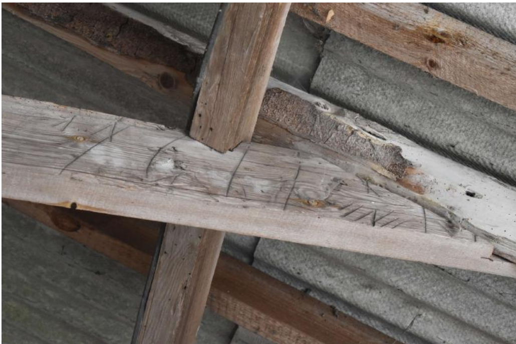
Photograph 38 Interior of Pond Barn, detail of Baltic Timber mark on collar (building 8). Photograph taken facing north-west.
