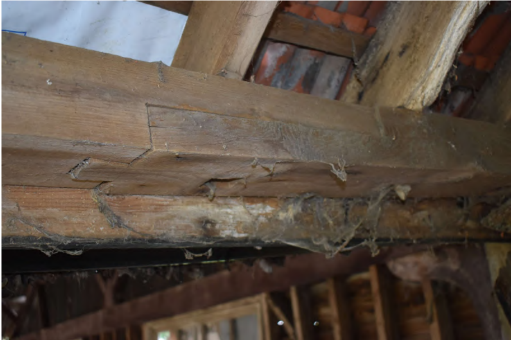
Photograph 46 Interior of Field Barn, detail of scarf-joint on the south-east wall-plate (building 10). Photograph taken facing south-east.
