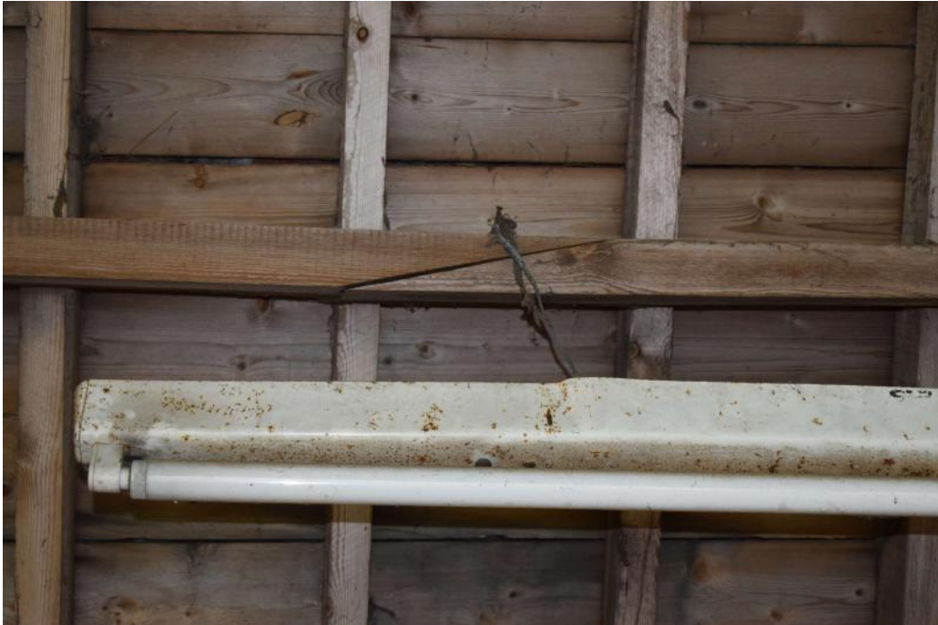
Photograph 19 Interior of Bailey Barn, detail of scarf-joint in purlin on north-east roof pitch (building 2). Photograph taken facing north-east.
