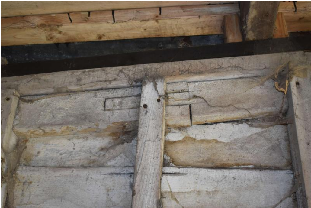
Photograph 27 Interior of Road Barn, detail of side-bridled scarf-joint in the south-eastern wall-plate (building 5). Photograph taken facing south-east.
