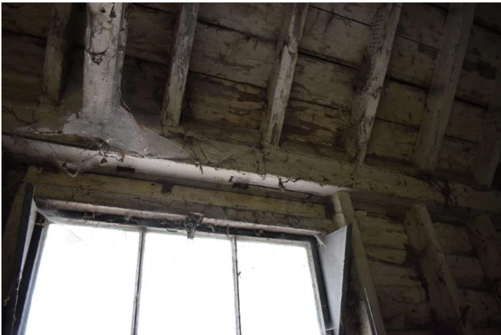
Photograph 25 Interior of Road Barn, detail of side-halved scarf-joint (building 3). Photograph taken facing north north-west.
