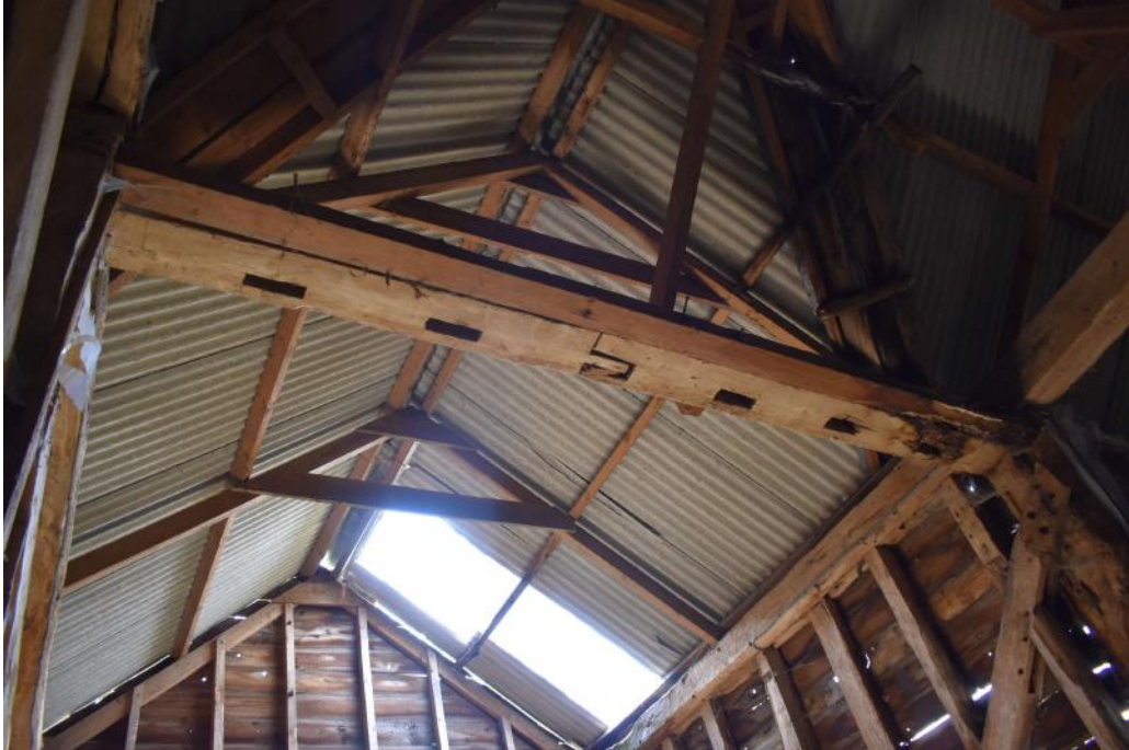
Photograph 12 Interior of Bailey Barn, detail of empty mortices and scarf-joint in south-east wall-plate of bay 3 (threshing barn). Photograph taken facing south south-east.
