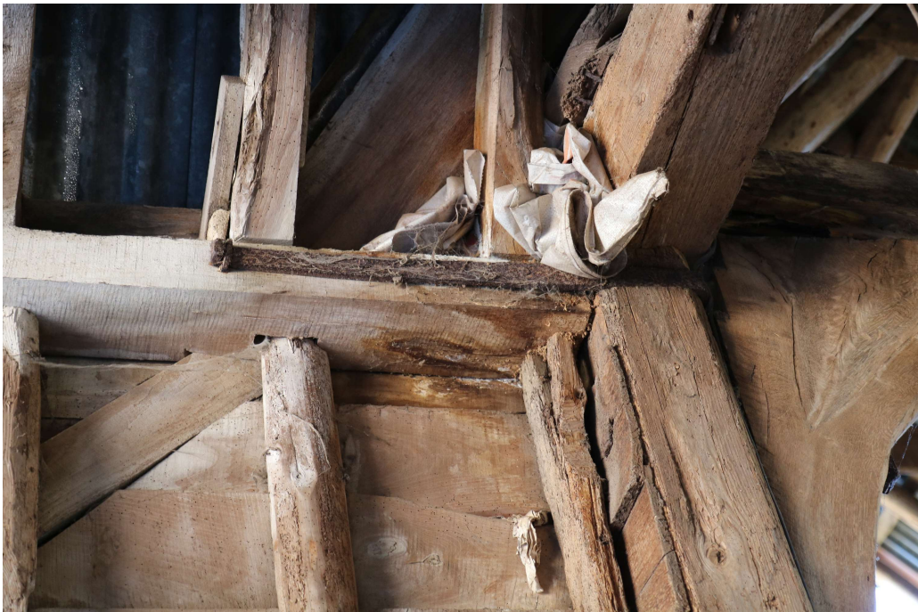
Photograph 19 Detail of iron strap in eastern wall-plate of midstrey of threshing barn. External weatherboarding visible adjacent to the right-most stud. Photograph taken facing east.
