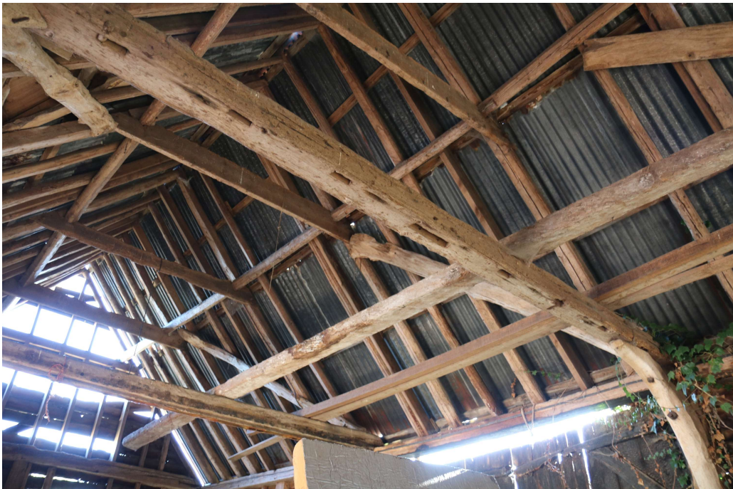
Photograph 11 Detail of reused tie-beam between bays 1 and 2 of threshing barn. Photograph taken facing south-east.
