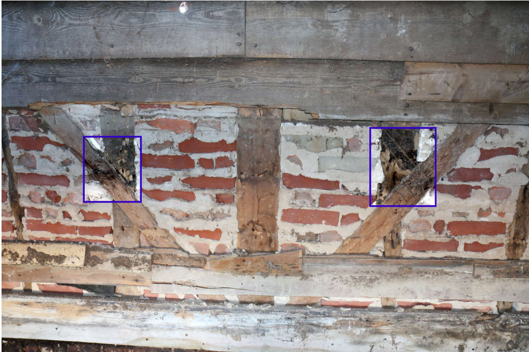
Photograph 36 Detail of 'III' and 'IIII' carpenter's marks in northern wall of bay 3 of threshing barn (seen in lean-to 2). Photograph taken facing south south-east.
