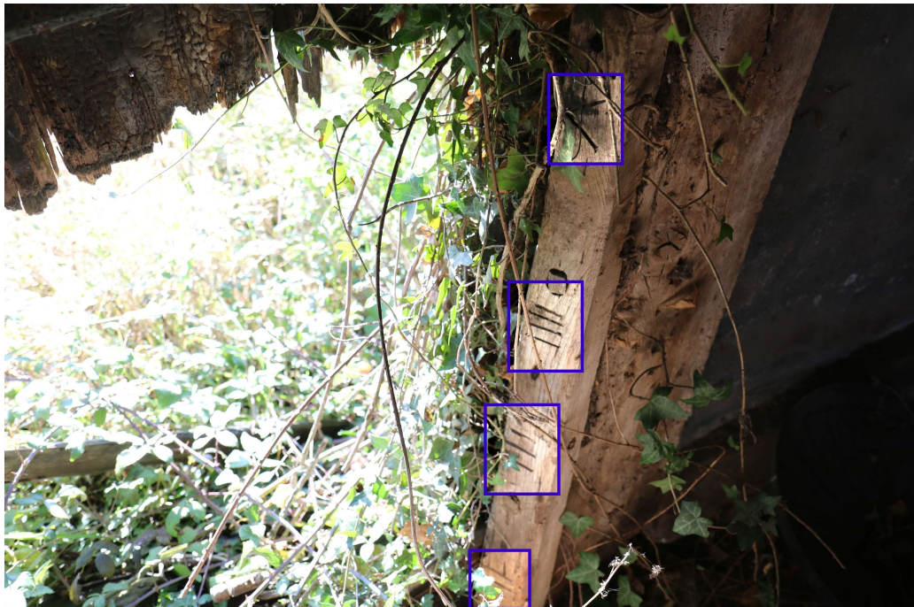
Photograph 16 Detail of carpenter's marks on timber adjacent to door in bay 2 of threshing barn. Photograph taken facing south south-west.
