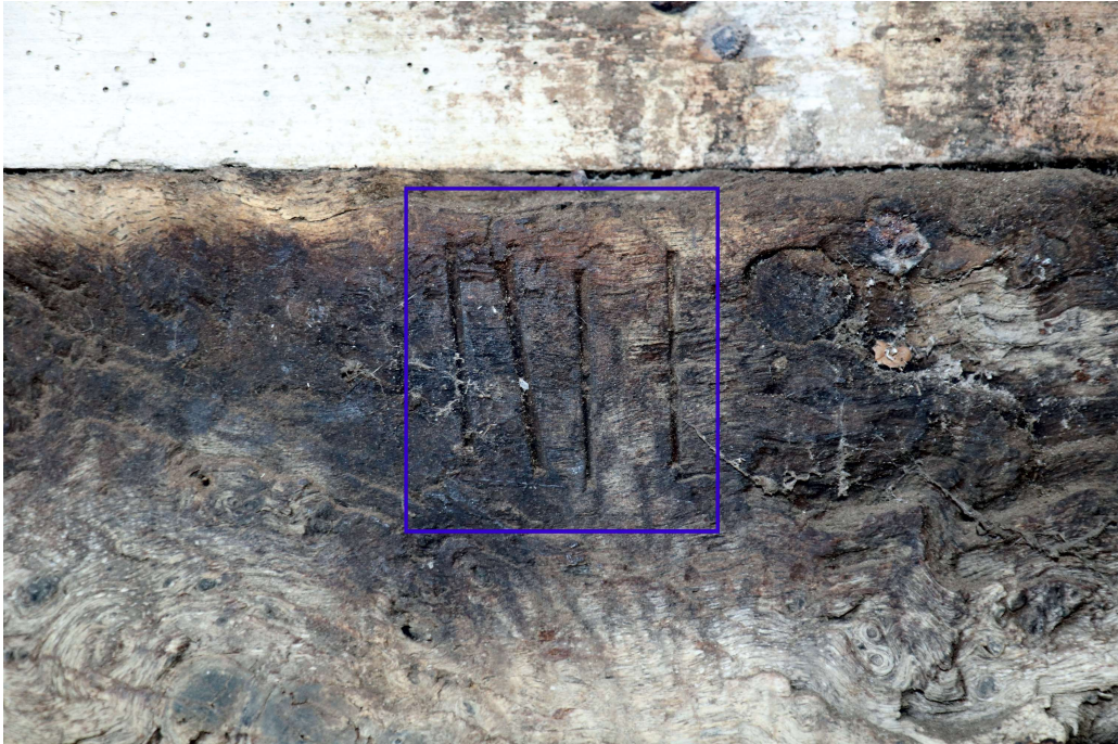
Photograph 24 Detail of carpenter's mark in northern sill-beam of bay 1 of four-bay building A. Photograph taken facing north north-west.
