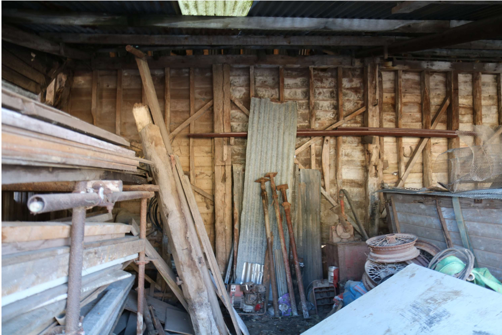
Photograph 12 Detail of exposed timber-frame of threshing barn in lean-to 1. Photograph taken facing south.
