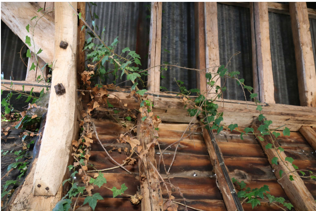
Photograph 14 Detail of wall-plate scarf joint in southern wall of bay 1 of threshing barn. Photograph taken facing south.
