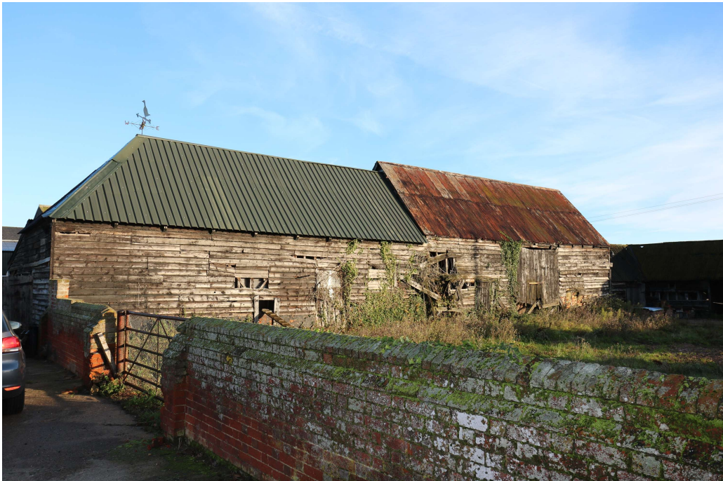
Photograph 9 Southern elevation, boundary wall visible in the foreground. Photograph taken facing north-east.
