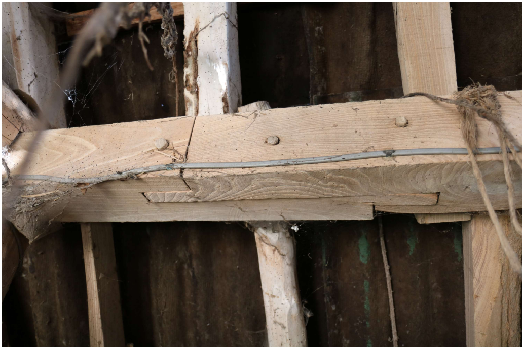
Photograph 32 Detail of scarf-joint in eastern arcade-plate of six-bay building (bay 3). Photograph taken facing east north-east.
