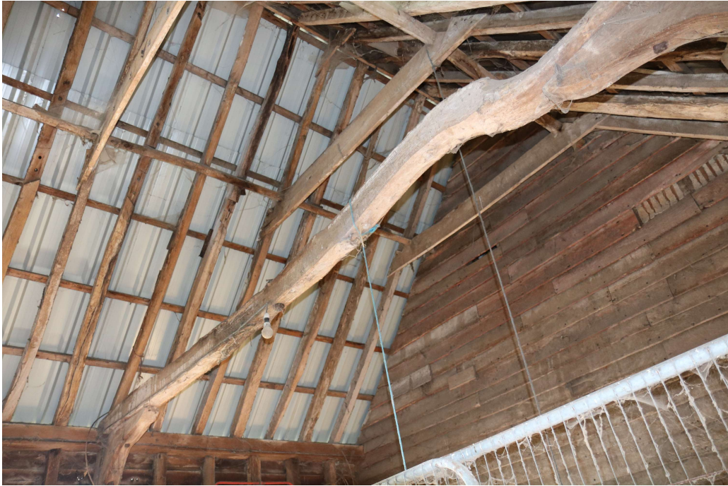
Photograph 20 Detail of roof construction of four-bay building A. Photograph taken facing south-west.
