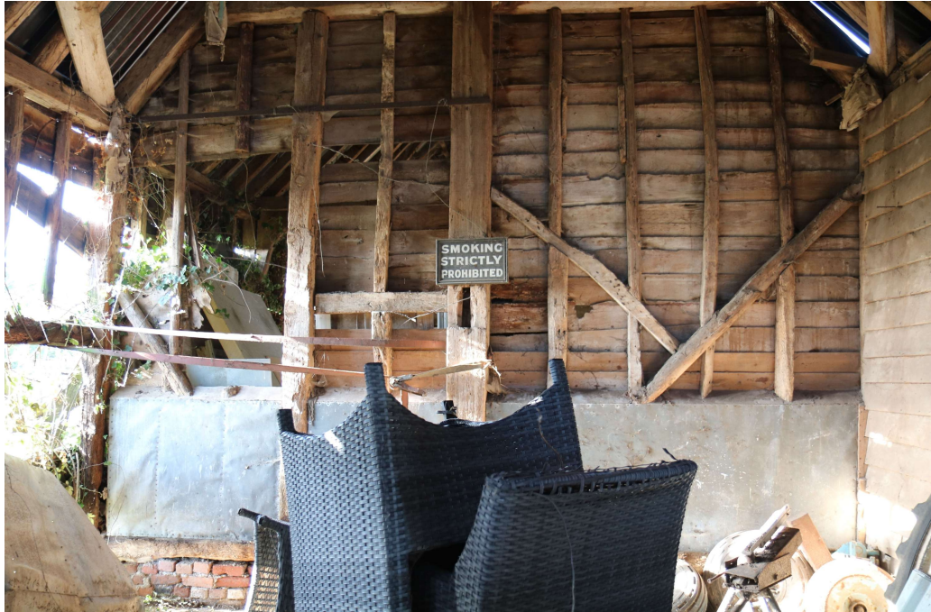
Photograph 15 Western wall of bay 1 of threshing barn. Photograph taken facing west south-west.
