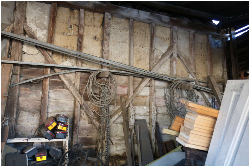
Photograph 21 Detail of exposed timber-frame of four-bay building A in lean-to 1. Photograph taken facing south.
