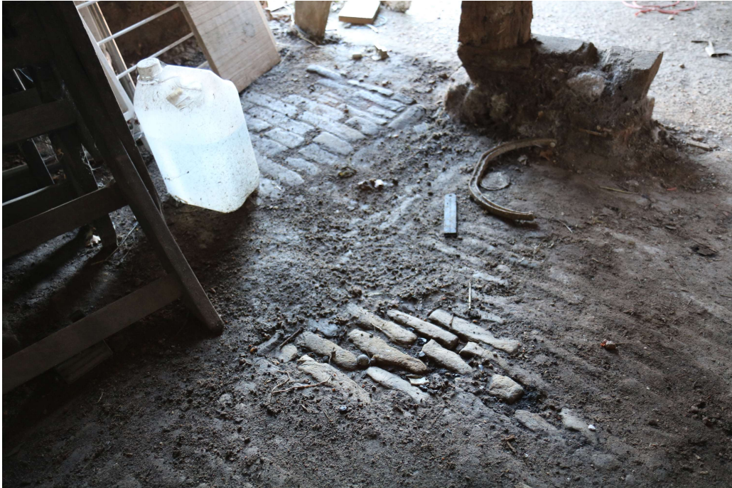
Photograph 26 Detail of brick floor in bay 1 of four-bay building A. Photograph taken facing north-west.
