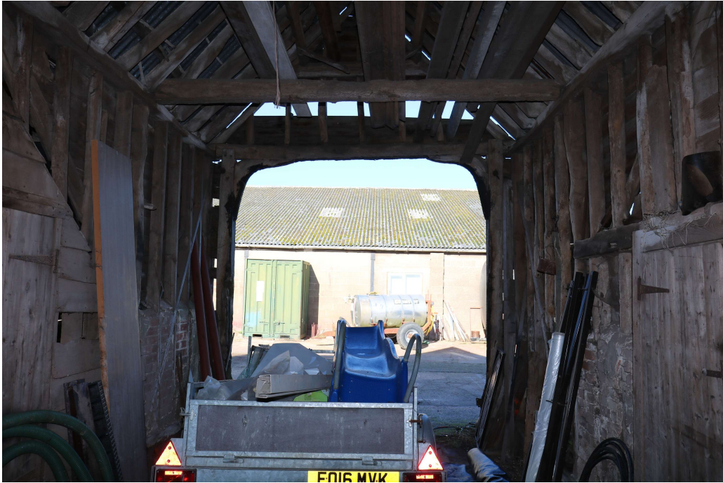
Photograph 18 Northern wall of midstrey of threshing barn. Photograph taken facing north north-west.
