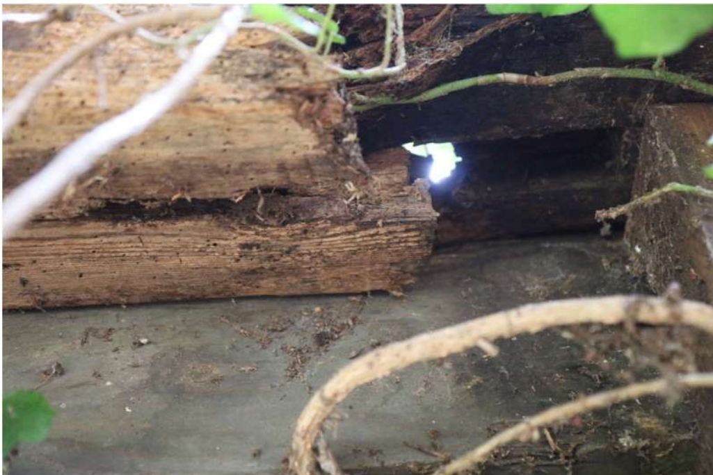
Photograph 23 Detail of possible scarf-joint in south-west wall-plate. Photograph taken facing south-west.
