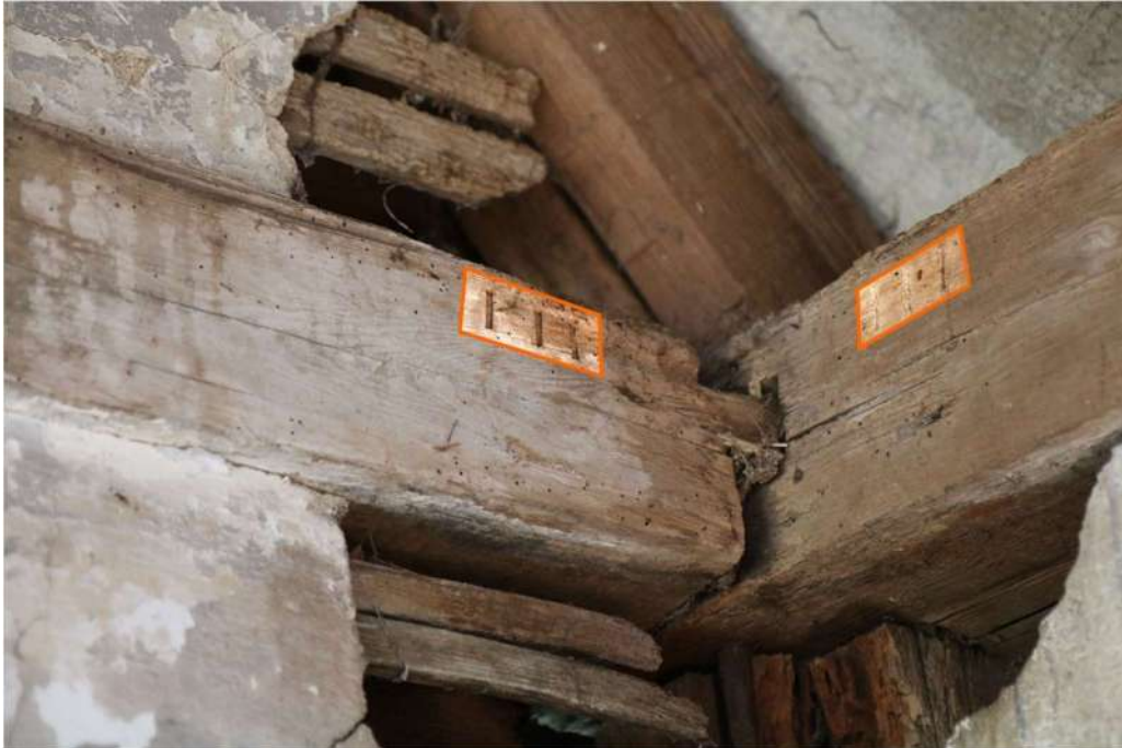
Photograph 22 Detail of carpenter's marks on wall-plate of store. Photograph taken facing south.
