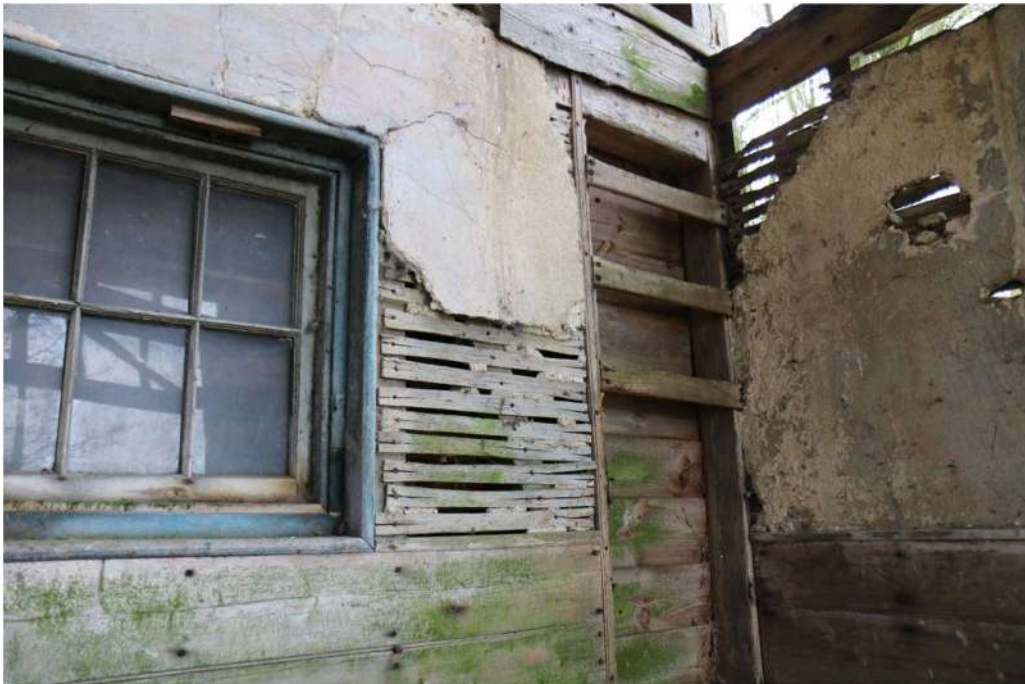
Photograph 17 Detail of exposed laths and ladder in the western corner of barn. Photograph taken facing west.
