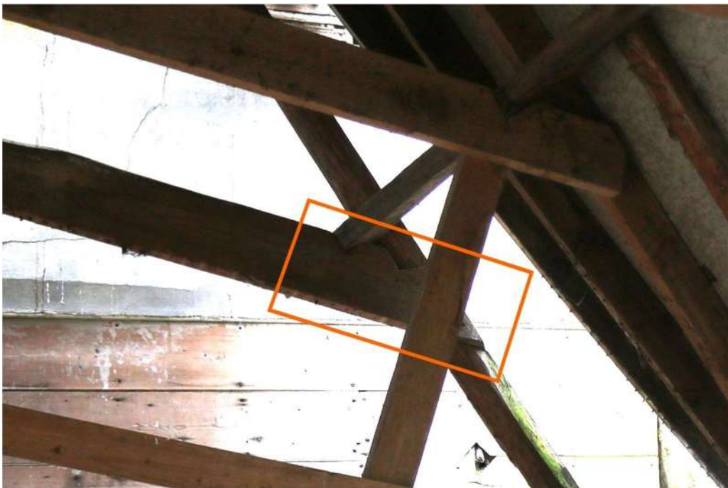
Photograph 19 Detail of lap-dovetail joint on collar in store. Photograph taken facing north.
