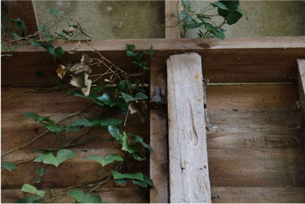
Photograph 16 Detail of pintle on post in south-west wall of barn. Photograph taken facing south-west.
