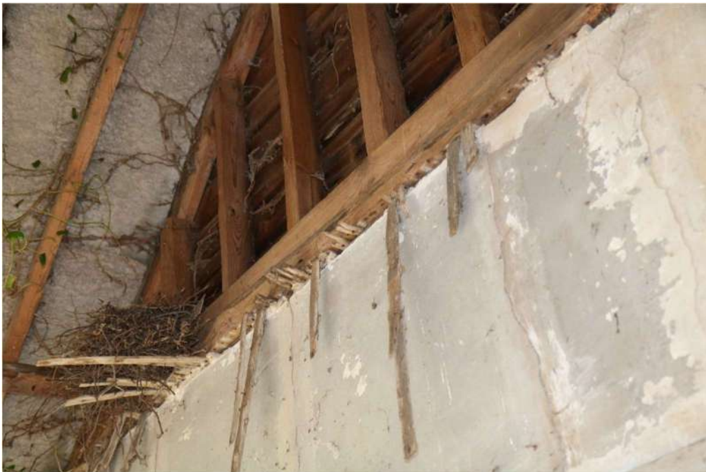
Photograph 21 Detail of remains of ceiling laths in store. Photograph taken facing east.
