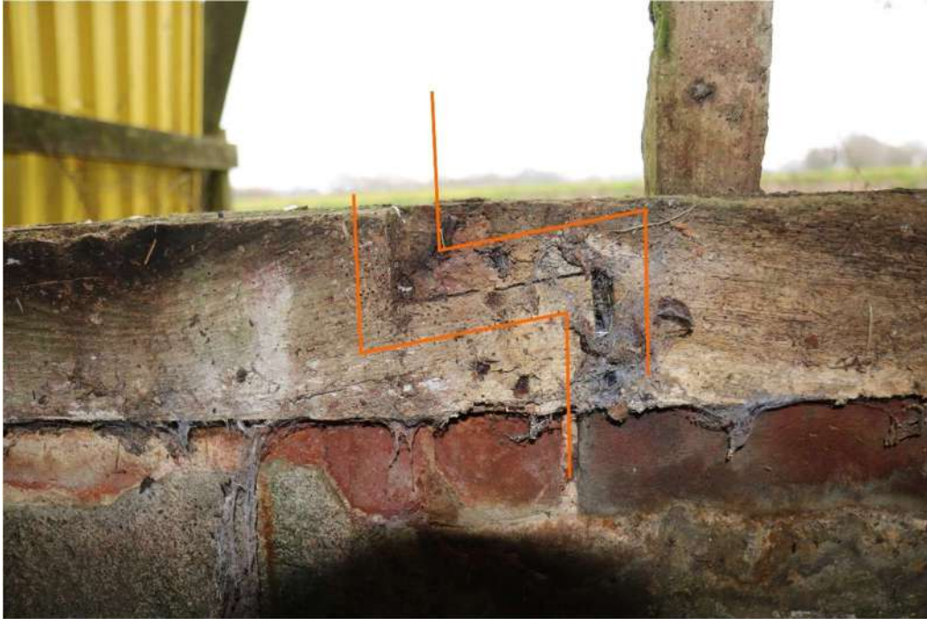
Photograph 12 Detail of scarf-joint in north-east sill-beam of barn. Photograph taken facing north-east.
