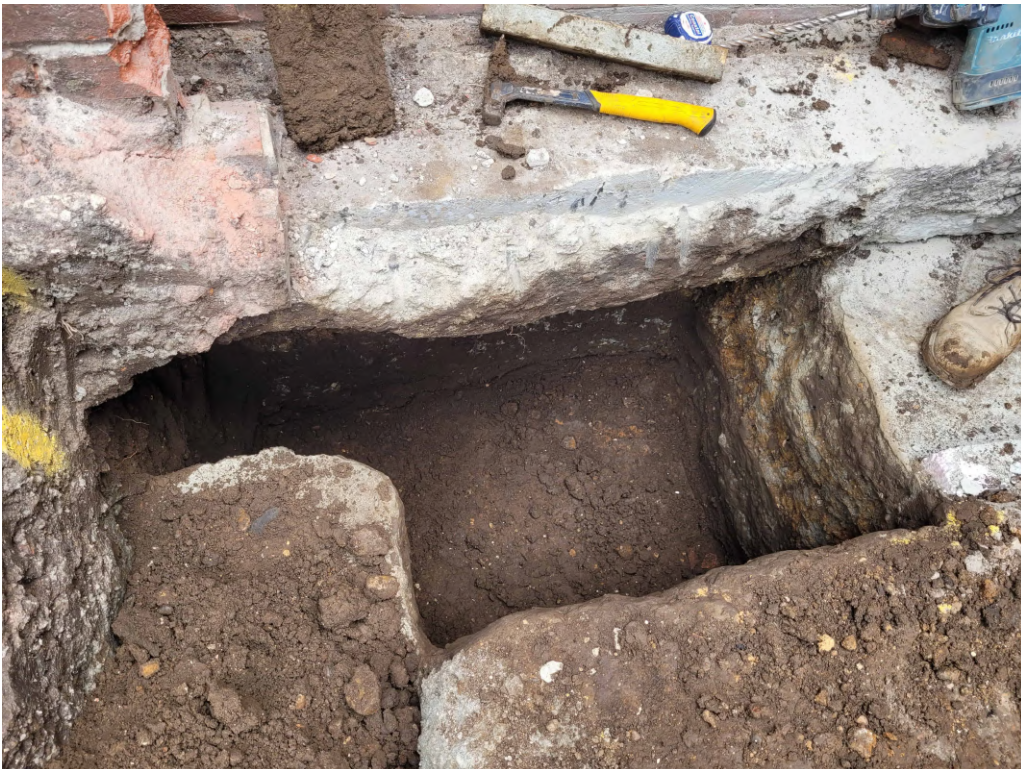
Photograph 4 Foundation trench showing excavation underneath the strip of concrete to the north of the site, looking north.
