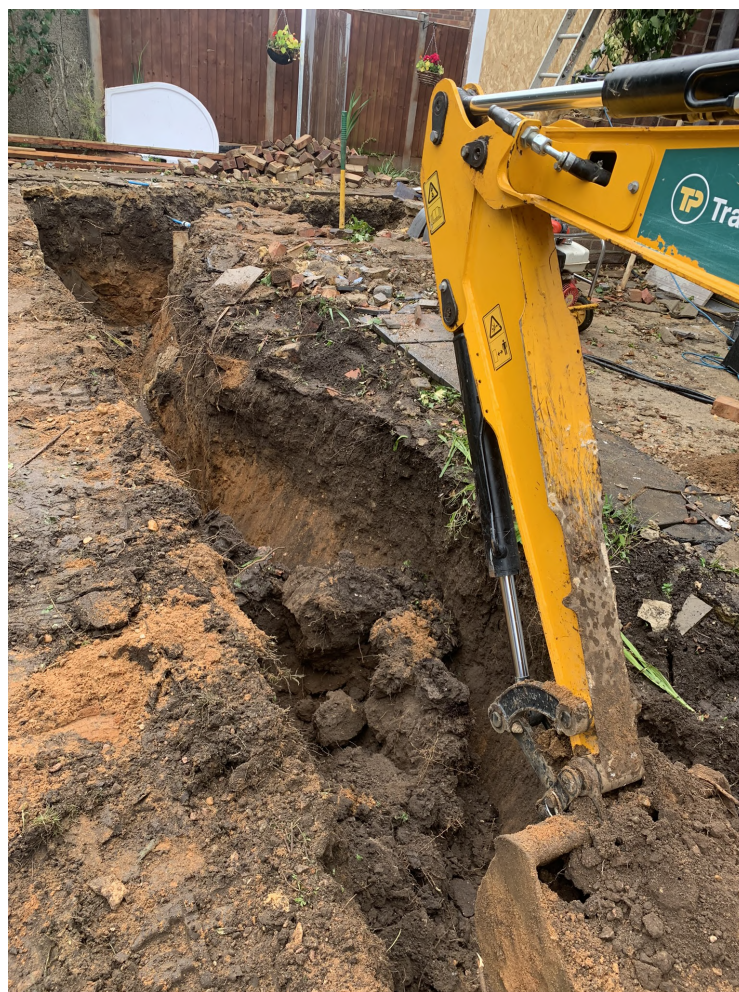
Photograph 2 Trench collapse, looking north.
