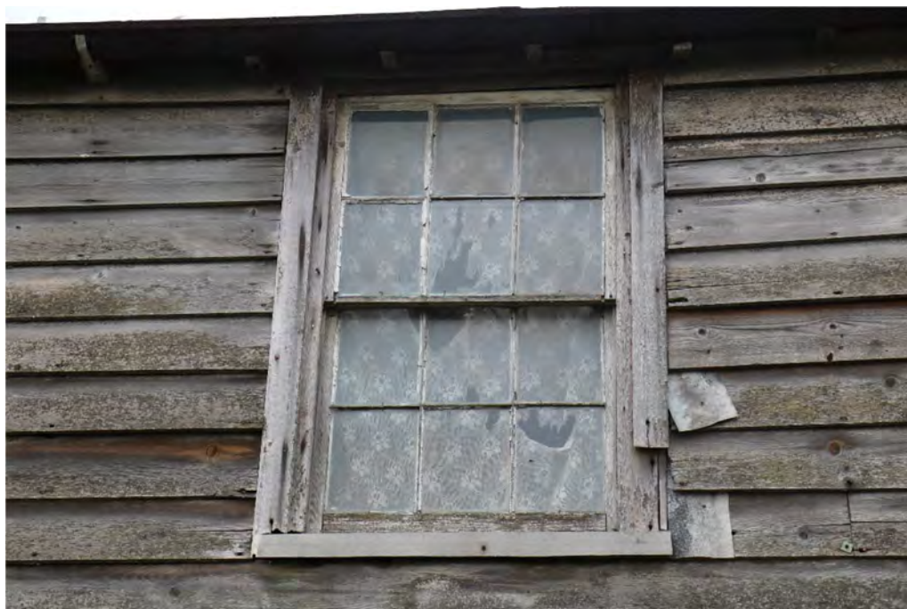
Photograph 7 First floor window on western elevation of building B. Photograph taken facing east.
