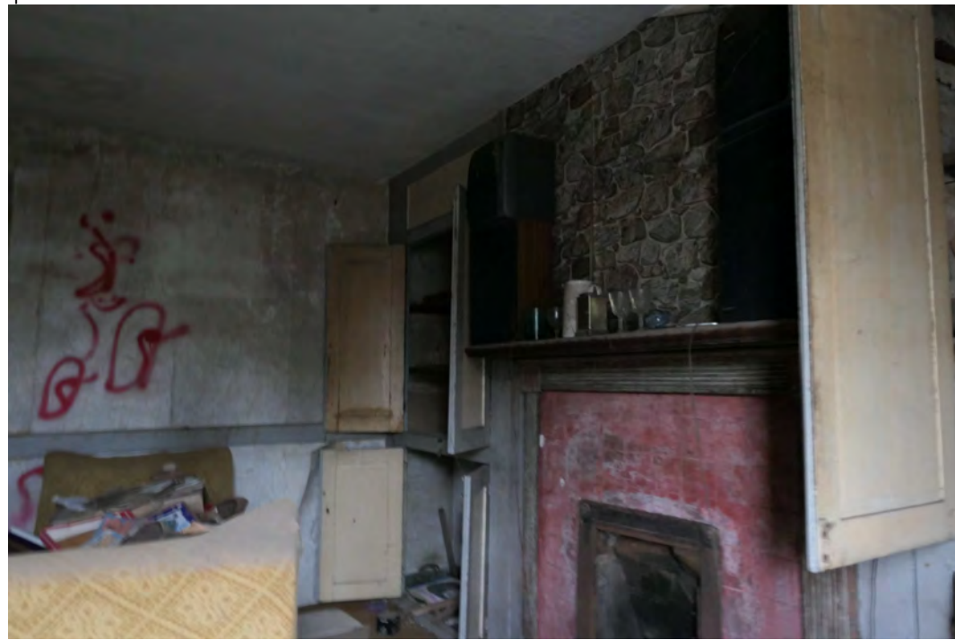
EEX60394_PhotoGraph_042 Interior of room 2 on the ground floor in building A. Photograph taken facing north-west.
