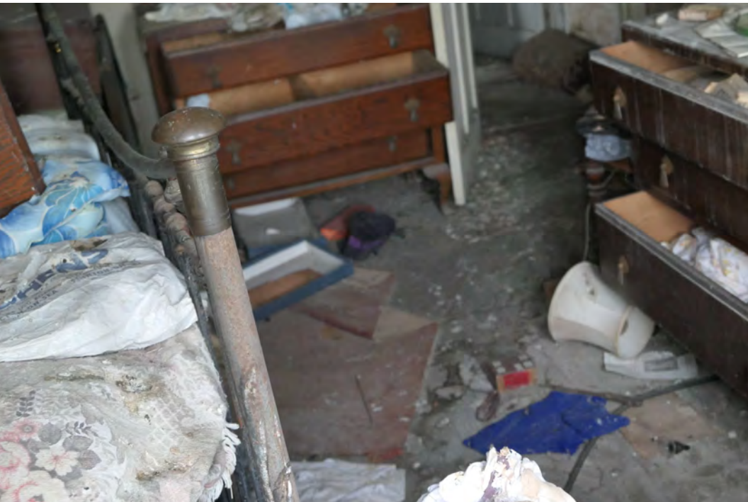
EEX60394_PhotoGraph_051 Close up interior shot of room 4 on the first floor in building A. Photograph taken facing north-west.
