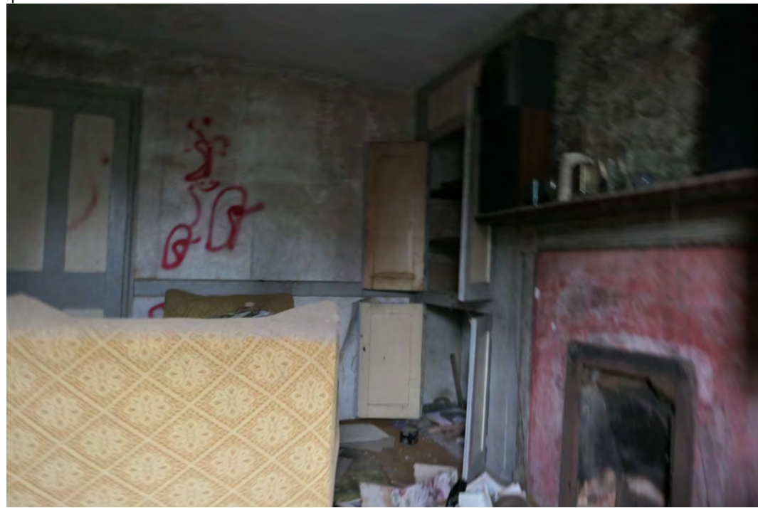
EEX60394_PhotoGraph_046 Ground floor window on northern elevation of building 2. Photograph taken facing south.
