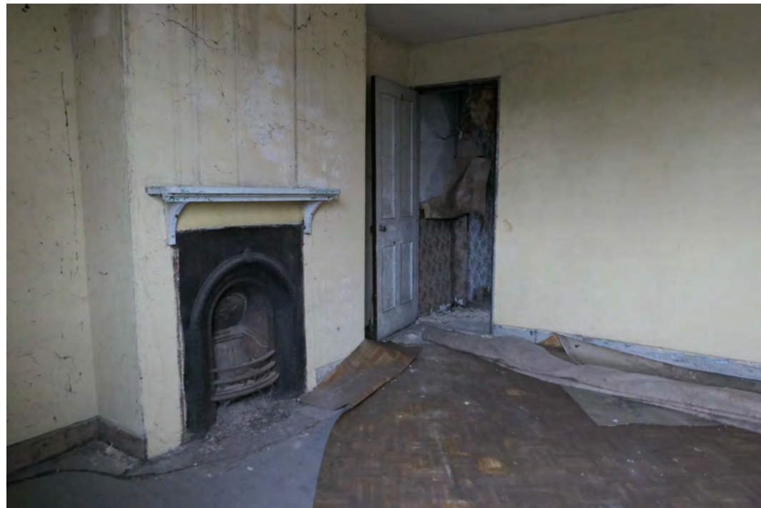
EEX60394_PhotoGraph_036 Interior of room 4 on the first floor in building B. Photograph taken facing south-west.
