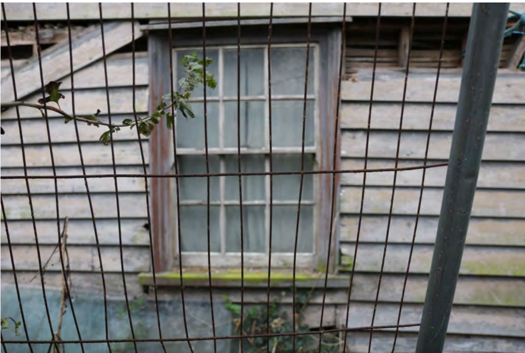
EEX60394_PhotoGraph_019 Ground floor window on northern elevation of building B. Photograph taken facing south.
