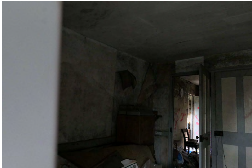
EEX60394_PhotoGraph_048 Interior of room 2 on the ground floor in building A. Photograph taken facing south-west.
