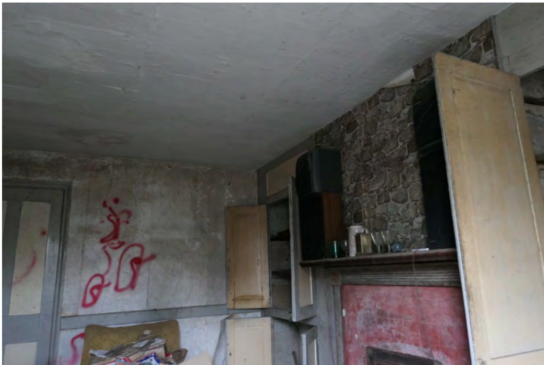
EEX60394_PhotoGraph_047 Ground floor window on northern elevation of building 2. Photograph taken facing south.
