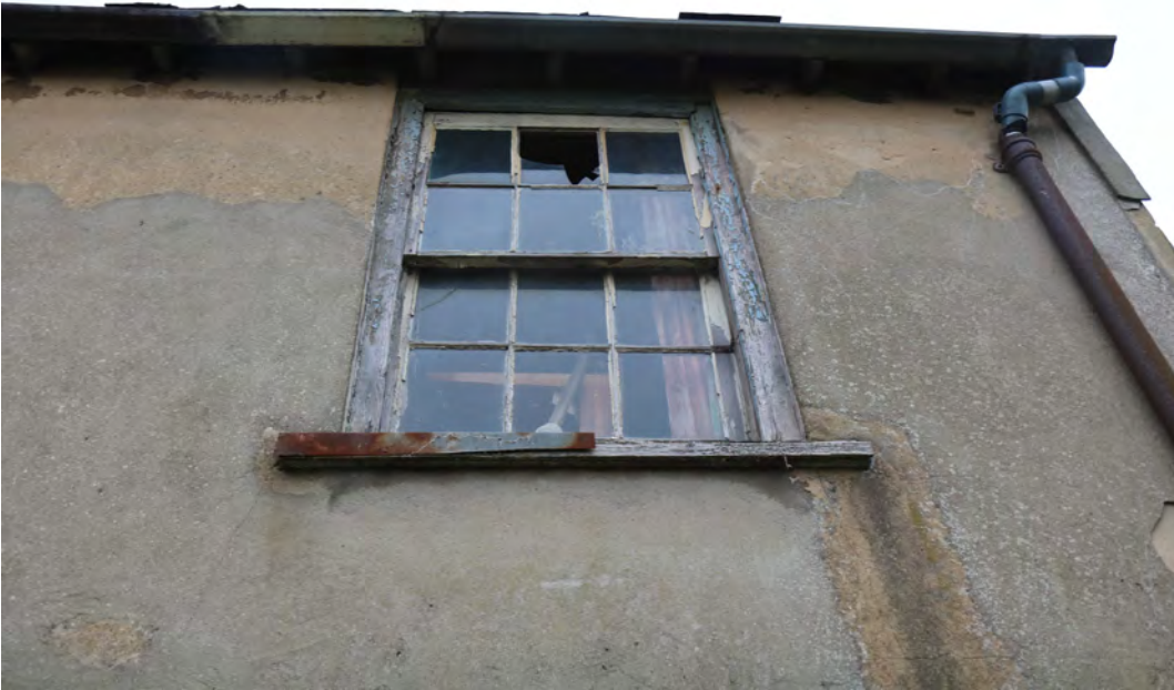
EEX60394_PhotoGraph_017 First floor window on western elevation of building A. Photograph taken facing east.
