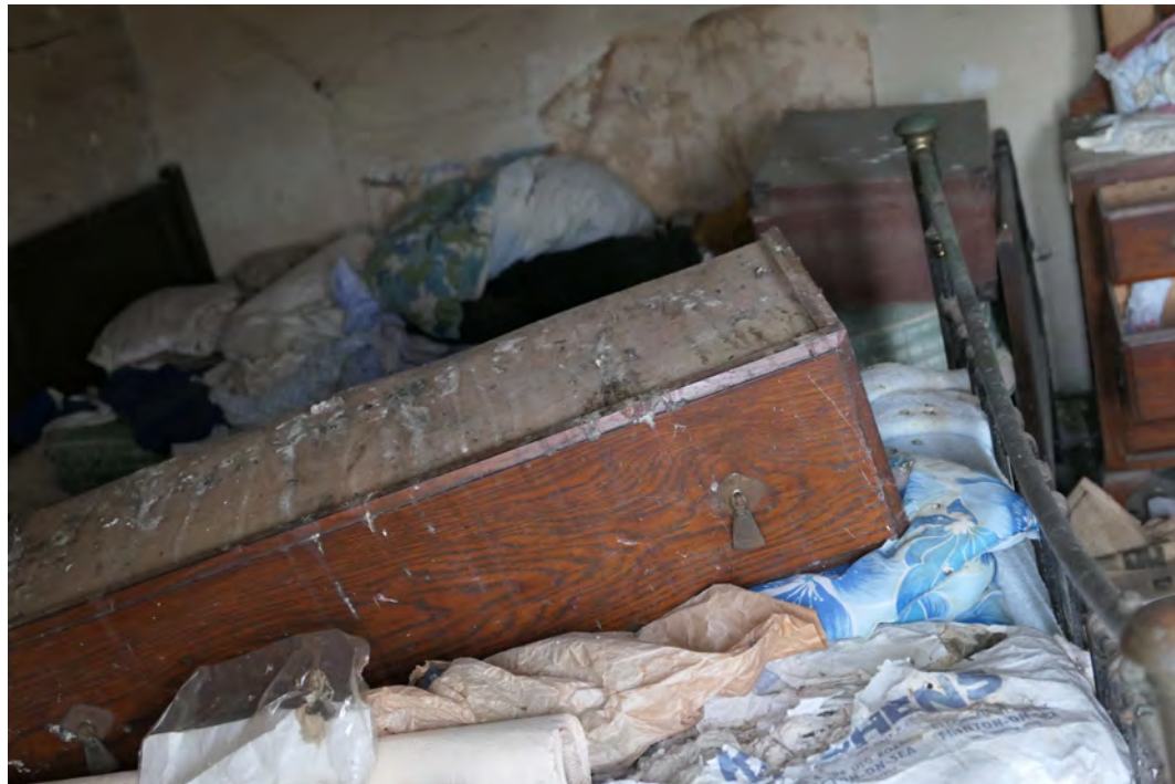
EEX60394_PhotoGraph_052 Detail of exposed timber-framing on northern elevation of building 2. Photograph taken facing south-west.
