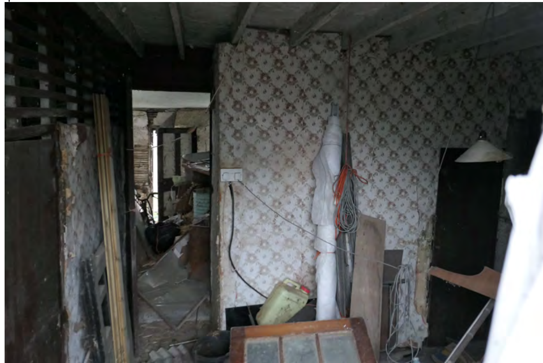
EEX60394_PhotoGraph_066 Interior shot of room 1 on the ground floor in building B. Photograph taken facing east.
