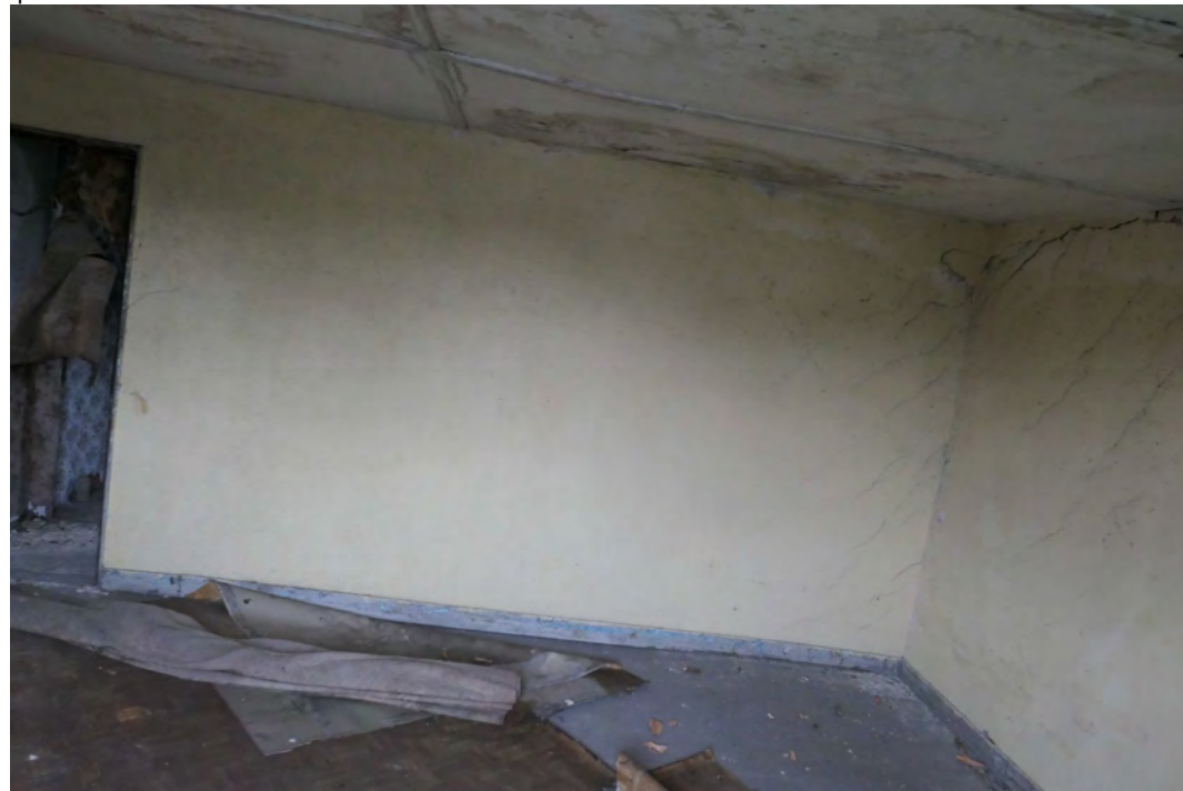
EEX60394_PhotoGraph_038 Interior of room 4 on the first floor in building B. Photograph taken facing north-west
