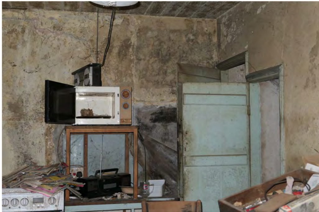
Photograph 10 Interior shot of room A1 on the ground floor in building A. Photograph taken facing north.
