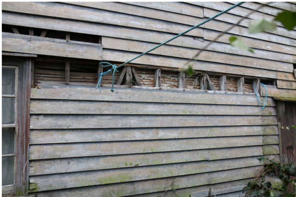
Photograph 9 Detail of exposed timber-framing on northern elevation of building B. Photograph taken facing south-west.
