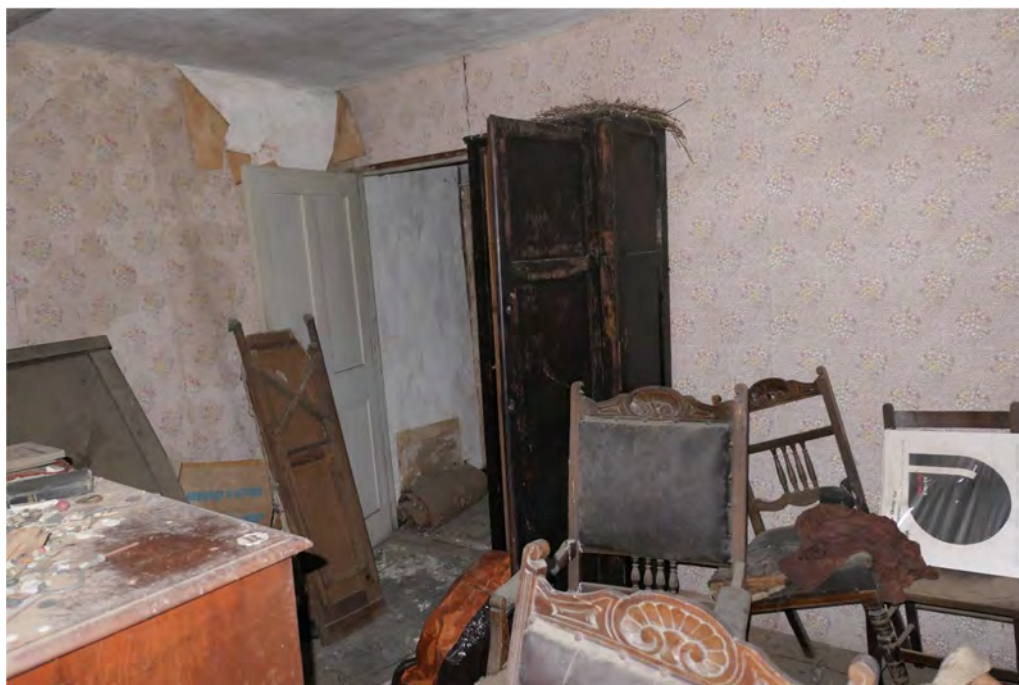
Photograph 12 Interior shot of room A3 on the first floor in building A. Photograph taken facing north-east.
