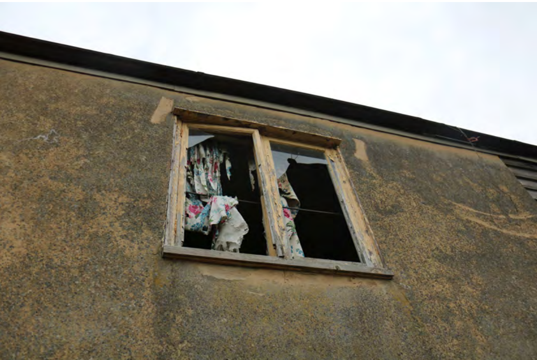
EEX60394_PhotoGraph_007 Ground floor window of building B on eastern elevation. Photograph taken facing west.
