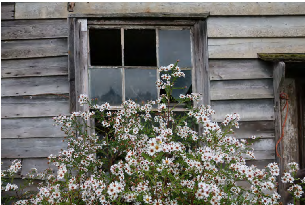
EEX60394_PhotoGraph_003 Ground floor window of building B on eastern elevation. Photograph taken facing west.
