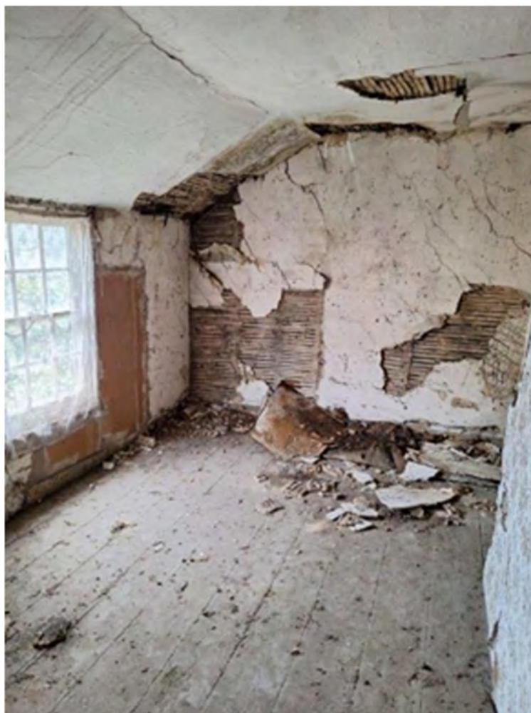
Photograph 16 Interior of room B3 in building B. Photograph taken facing north-west. (Photograph provided by client).
