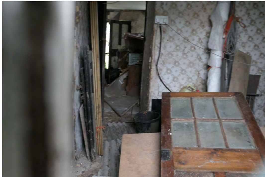
EEX60394_PhotoGraph_068 Interior of room 4 on the first floor in building 2. Photograph taken facing south-west.
