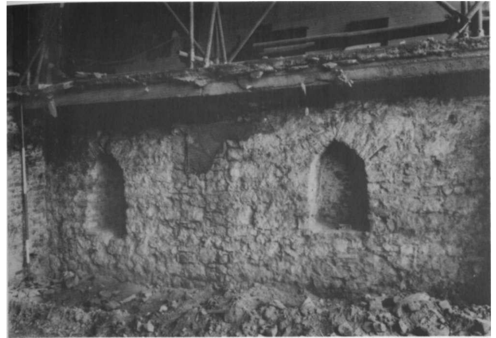
Thirteenth- or fourteenth-century cellar, built of peg-tile and reused Roman materials. Part of the original house bought by the Osbornes. Discovered in 1985 during rebuilding works.
